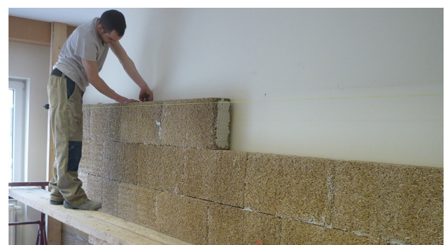
Figure 5 Acoustic interior insulation with hempcrete blocks for a school renovation (iso hemp.com)
