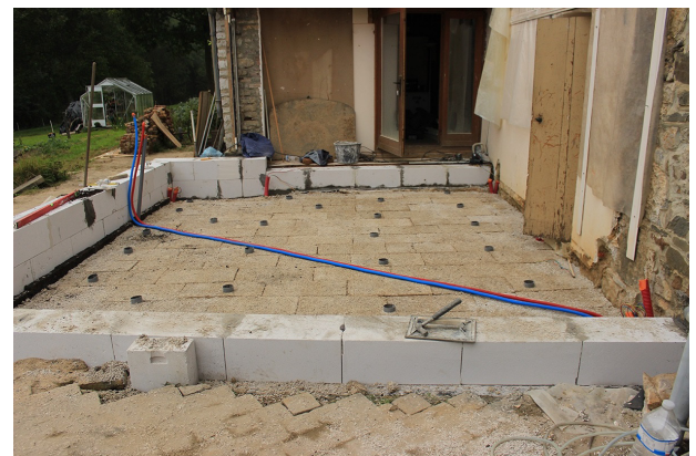
Figure 4 Floor isolation with hempcrete blocks and no adhesive agent in a detached house (iso hemp.com)
