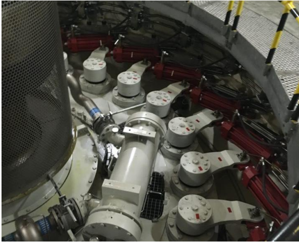
Figure 6: Wicket gates in turbine fieldtrip Cortes-La Muela
