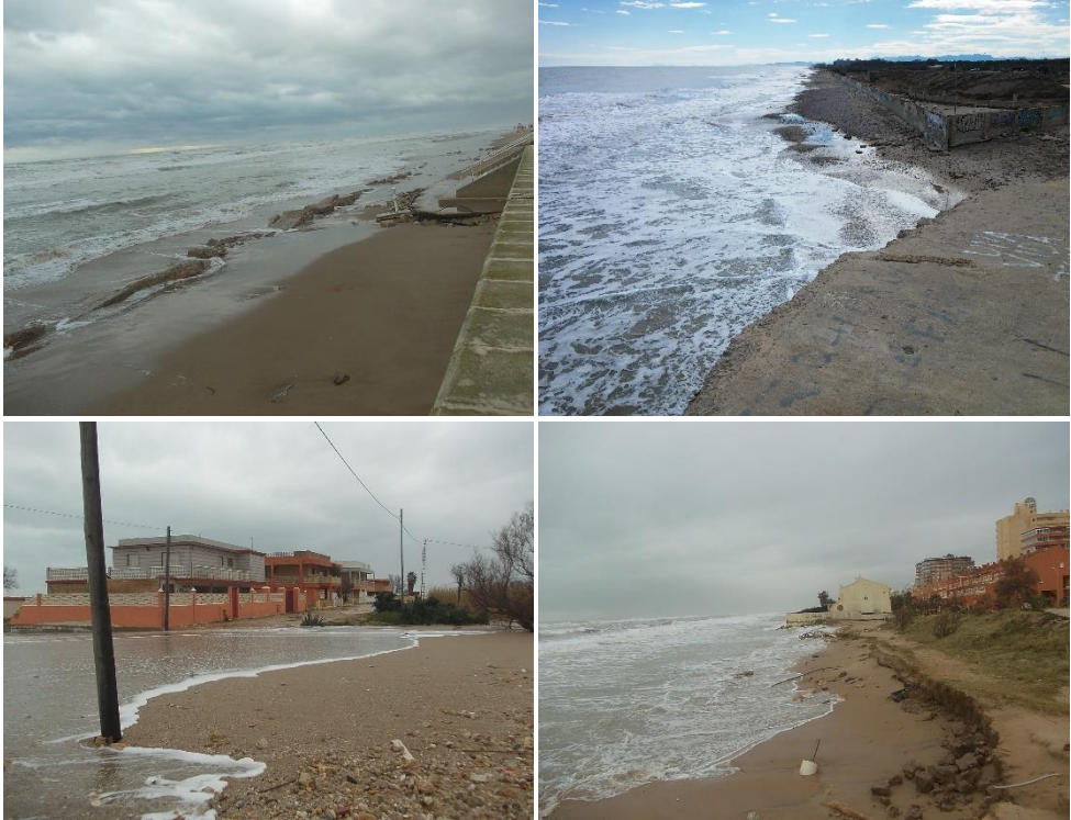
Fig. 6.4. Example of photos taken by the Valencian Coastal Demarcation employees on 23/01/2017. These show the damage caused by a major storm that hit the entire coast over the previous two days. The top photos are from the El Saler district and those below are from the municipality of Tavernes Blanques (all beaches to the south of the Port of Valencia).
