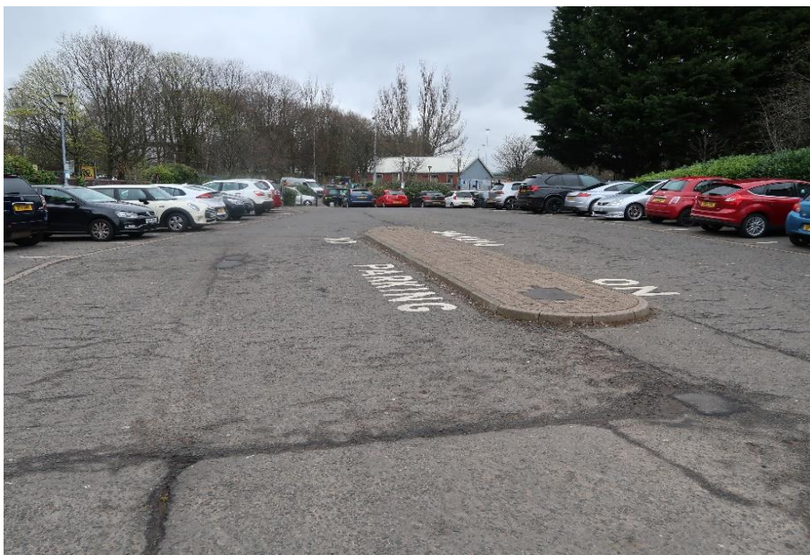
Figure 23. E4 Parking state
