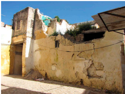
Figure 1. Precariousness of the buildings of the medina. Source: Photo taken by authors (2017).
