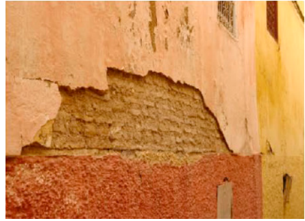
Figure 2. Water infiltration after restoration actions. Source: Photo taken by authors (2017).
