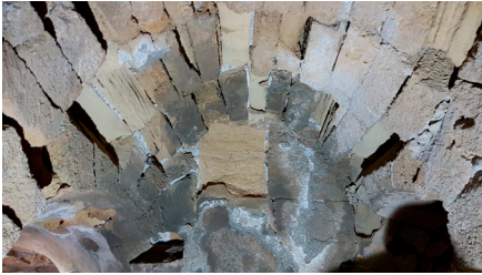
Figures 3-4. (top) Façade of Miagao Church; (bottom) Pulverization of stone and efflorescence on the vault at the second level of the right bell tower at the entrance from the choirloft. (Photo by Theo John Residilla, Dec. 2017).
