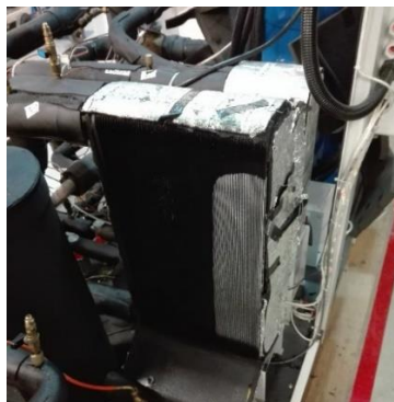
Figure 5. Ice deposit on outside of the BPHE
