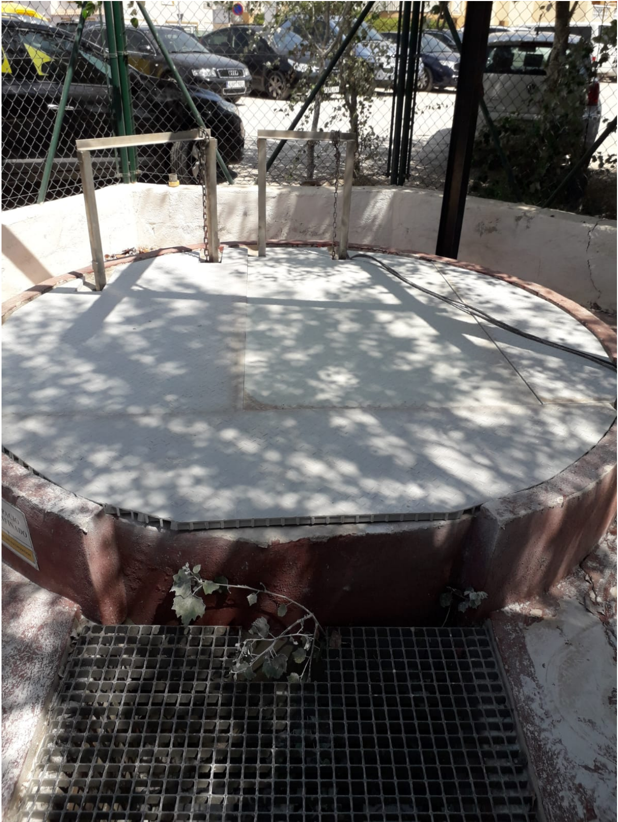
Figure 16: Pumping station 2 after sealing with metal plates on 7 August 2018.
