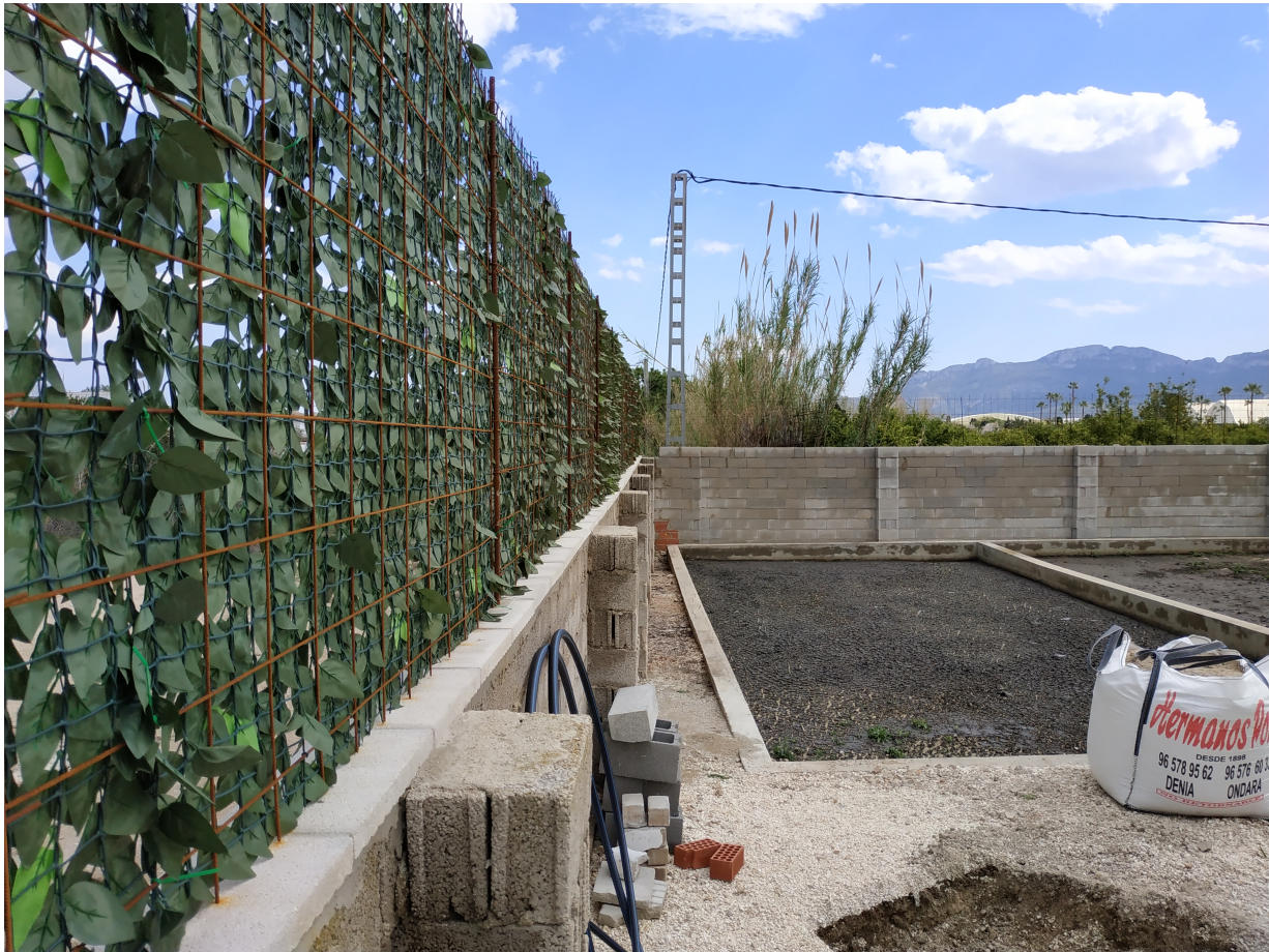
Figure 26: Picture of the sight protection fence built on top of the old low wall surrounding the WWTP-site (shot on 3 April 2019).
