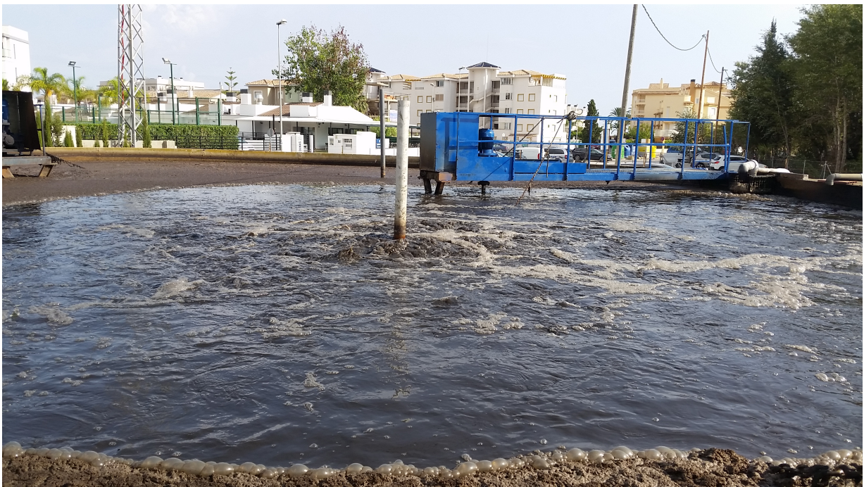
Figure 9: View of the new Venturi aeration system in action (shot taken on 5 September 2018).
