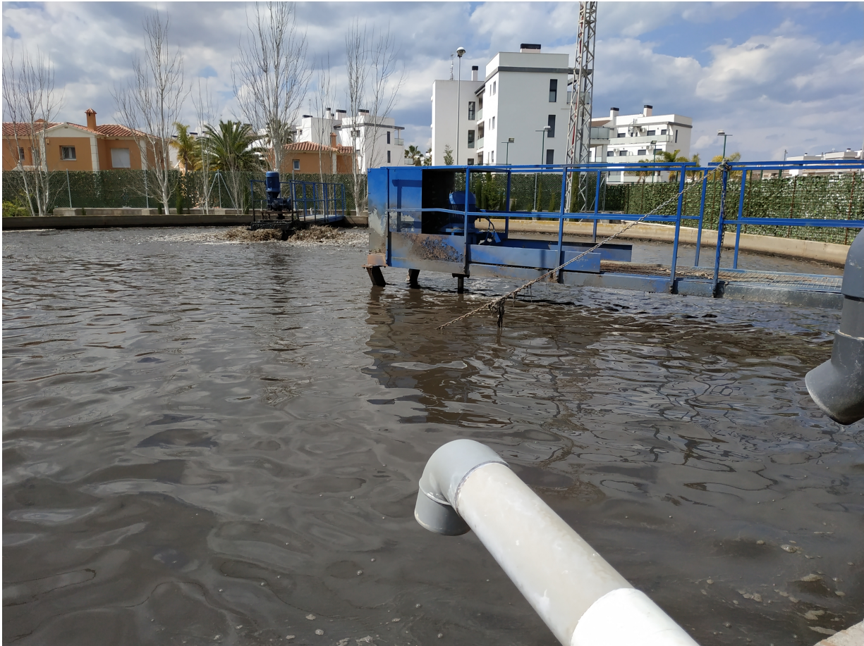
Figure 10: Snapshot of the old turbine aeration system in the bioreactor functioning during the visit of the WWTP Camping San Fernando when launching the second measurement campaign as of 3 April 2019.
