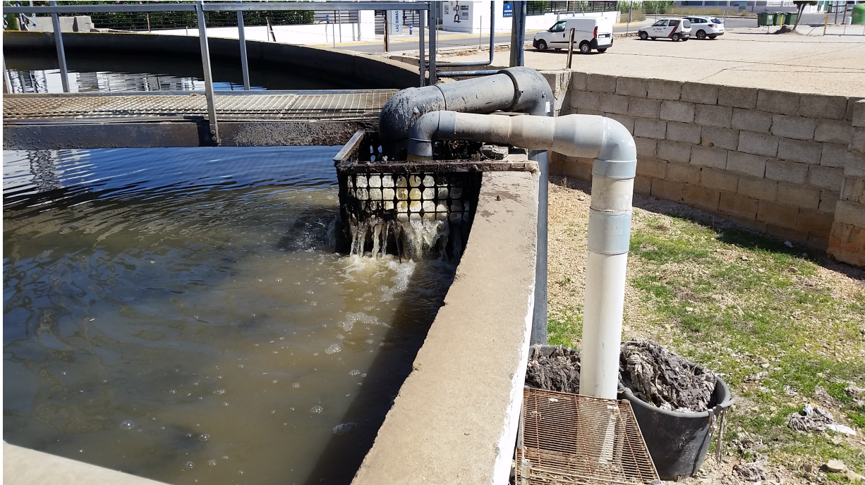
Figure 17: Picture of the coarse grate which was installed formerly at the outlet of the sewage system preventing chunky material from entering the primary biological reactor of the WWTP Camping San Fernando.
