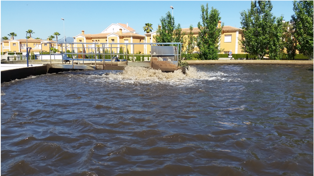
Figure 8: Photograph of the previous water surface turbines providing the oxygen supply of the bioreactor system with the aim to maintain it in an aerobic working state.
