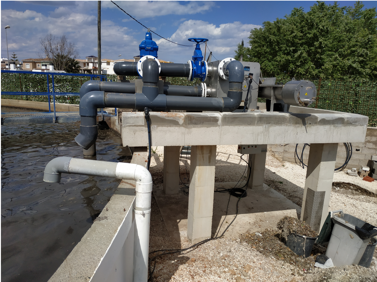
Figure 7: Closeup of the bioreactor entrance during the second measuring campaign 2019. As of spring 2019, it comprises of a new subterranean canalization entrance into the bioreactor with previous filtering via rotation sieves.
