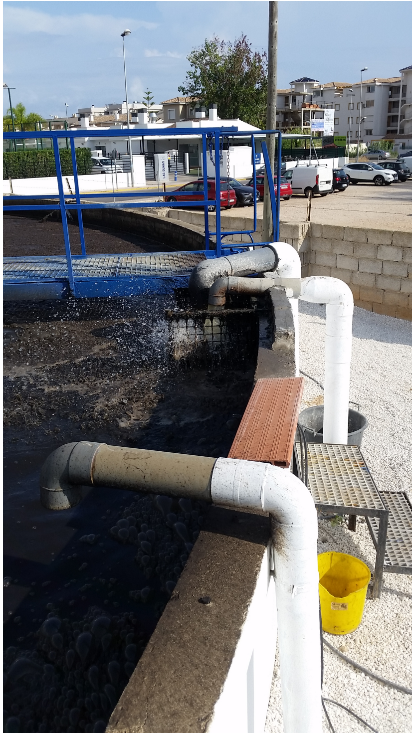
Figure 6: Photo of the bioreactor entrance during the first measuring campaign 2018 showing the active part of the pumping cycle (compare fig. 55 and 56) with a turbulent squirting waterfall, which was caused by the coarse grate installed directly underneath the pipe outlet.
