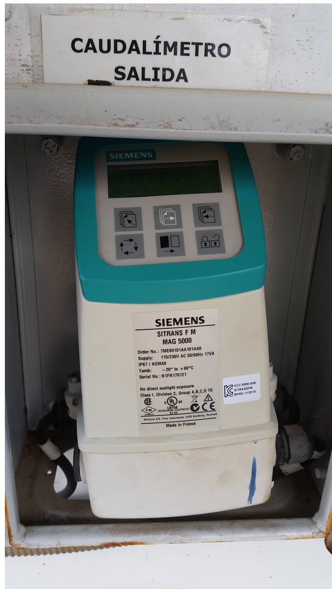
Figure 43: Photo of the fixedly installed volume flow meter which allows for reading off the currently accumulated volume outflow of the entire WWTP complex in cubic meters.
