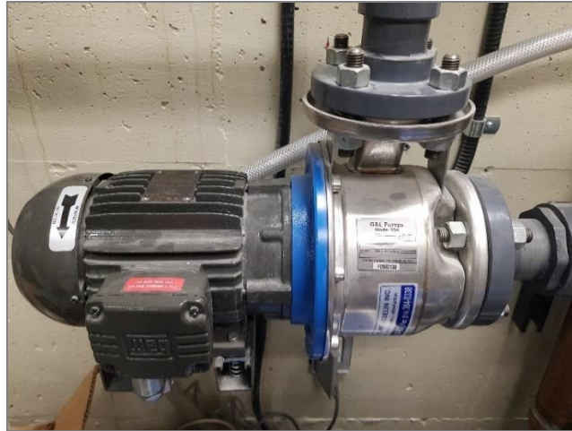
Figure 16: Pump water of the water tunnel
