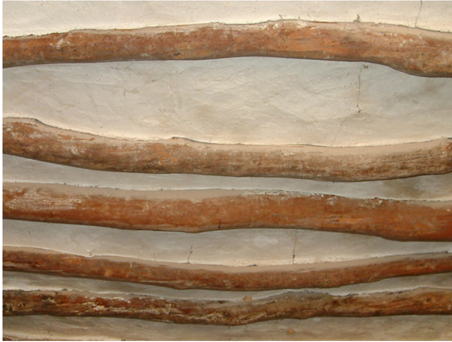
Figure 4. Twisted joists used as structural element in a homestead near Elda (Alicante)
