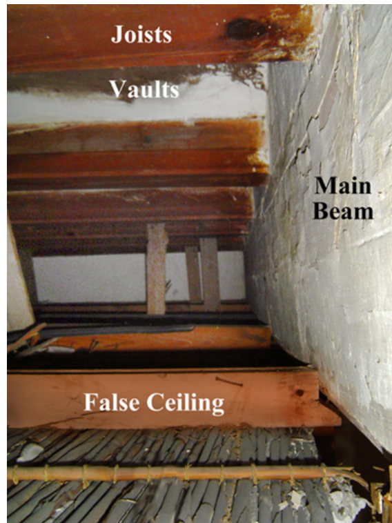
Figure 5. Hanged false ceiling structure made with timber frames, reeds panels and a plaster finishing underneath, School of Theology, Valencia, built around 1829-1853
