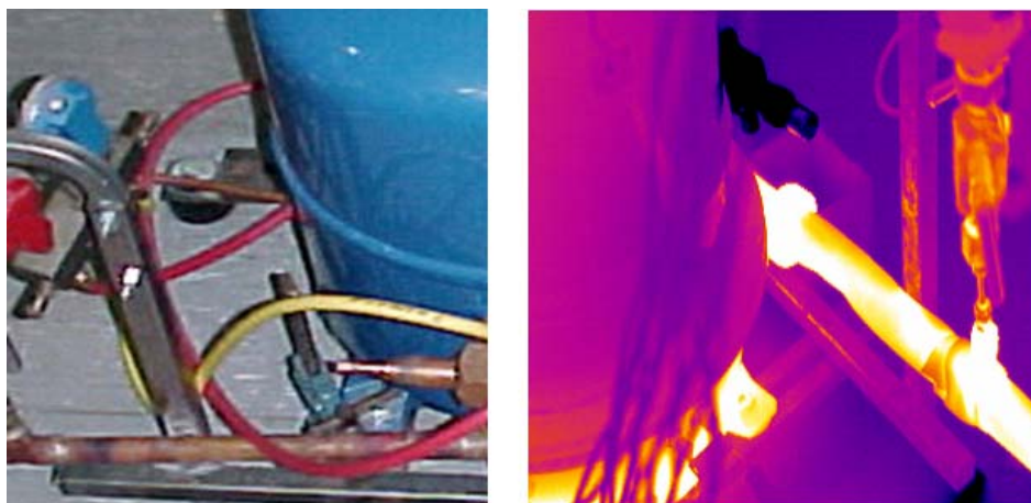
Figure C.3: Visual and infrared images of the outlet pipes of the compressor.
