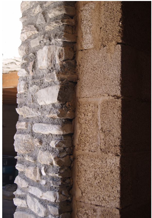
Figure 6. Re-qualification of a vertical closure by affixing a masonry of bricks and mortar in hemp and lime with the aim of increasing the thermal performance of the wall (source: Edilcanapa).
