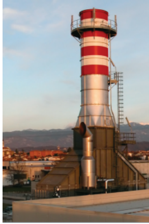
Figure 4: Once-through steam generator used in Gorizia Combined cycle Power Plant [12].
