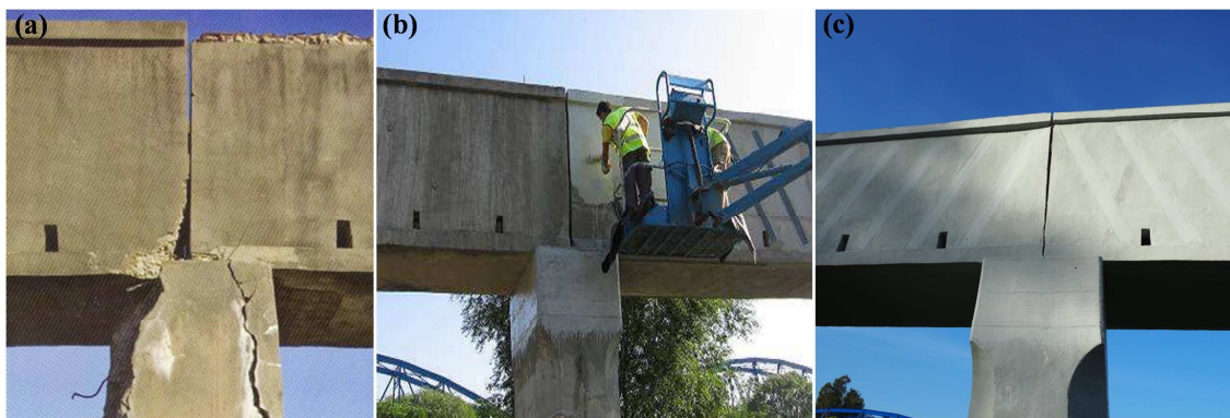
Fig 4: Tempul Aqueduct renovation works. (a) Before renovation, (b) Application of protective coating, (c) the aqueduct in October 2015, seven years later. Source: (a) and (b) COMPOSAN, (c) I. Paya-Zaforteza.
