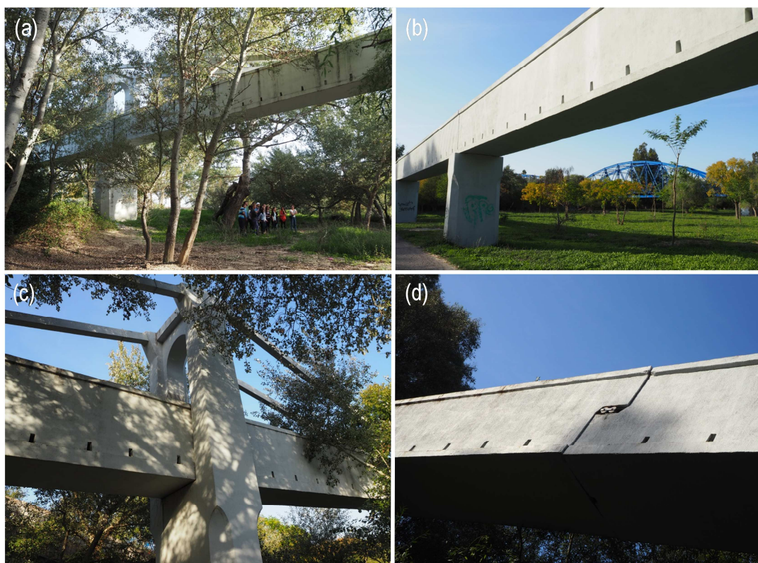
Fig 1: Current state of the Tempul Aqueduct: (a) General view. (b) Approaches. (c) Detail of the pylon. (d) Joint between the simply-supported and cantilevered spans. Pictures by Ignacio Paya-Zaforteza.
