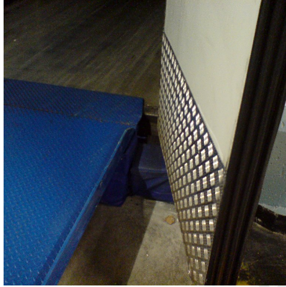
Figure 6: Contact between the back of the truck door and the dock door.
