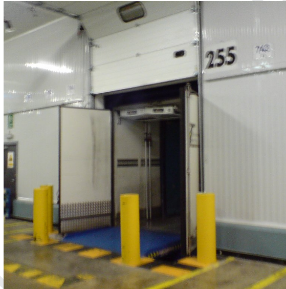
Figure 4: View of inflatable dock from inside the warehouse
