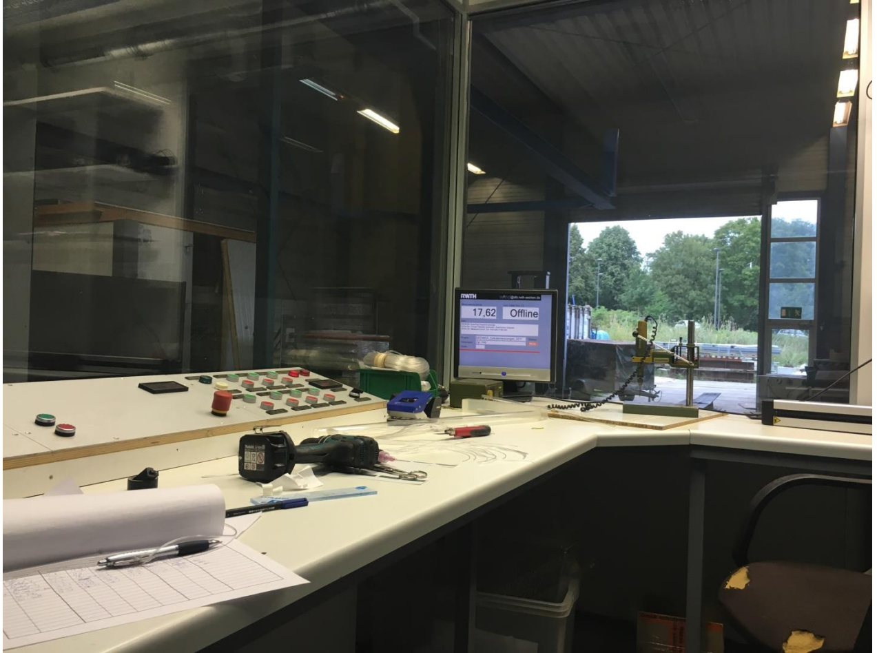
Figure A.9 control cubicle
