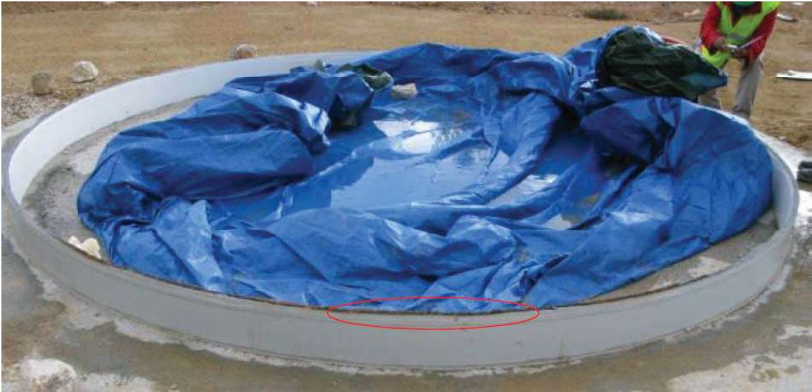
Fig. 4. View of the section in which the failure began
