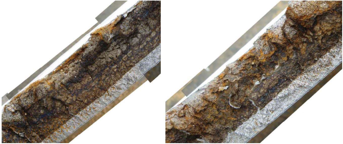
Fig. 7. Detail of the broken flange section
