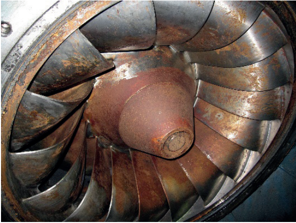
Figure 4: Mechanical disassembly of the hydroelectric group turbine due to predictive maintenance analysis (vibration and cavitation analysis) (Enel Green Power-Endesa Generation).
