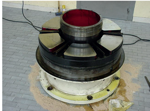
Figure 2: Assembly work of oil injection circuit to the pivot bearing of the hydroelectric group due to redesign by preventive maintenance analysis (Enel Green Power-Endesa Generation).
