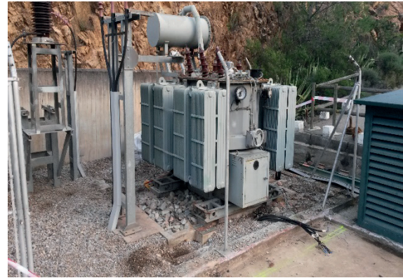
Figure 3: Power transformer replacement work due to predictive maintenance data analysis (dielectric oil analysis) (Enel Green Power-Endesa Generation).
