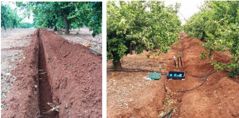
Fig. 3. Detail of the work for the installation of the surface and subsurface drip irrigation system.
