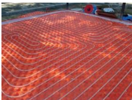
Figure 26. Example of a radiant floor. Source: Google Images.
