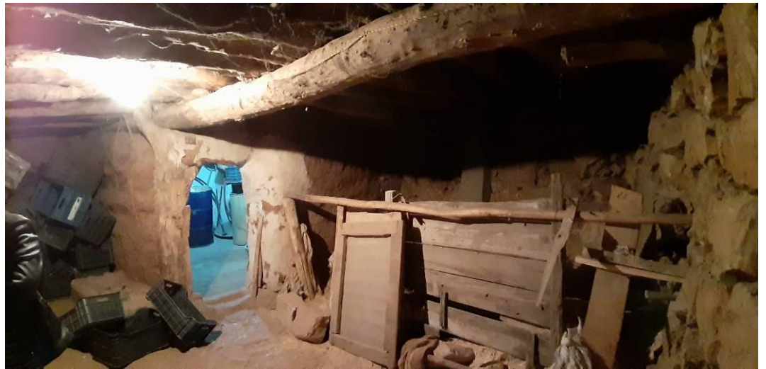
Figure 149 wall opening connecting space "1" and "2" which is the stable. Some concrete plaster patches are used over the mud and straw plaster. The door connecting both spaces is almost 90 x 165 cm source: Author (2018)
