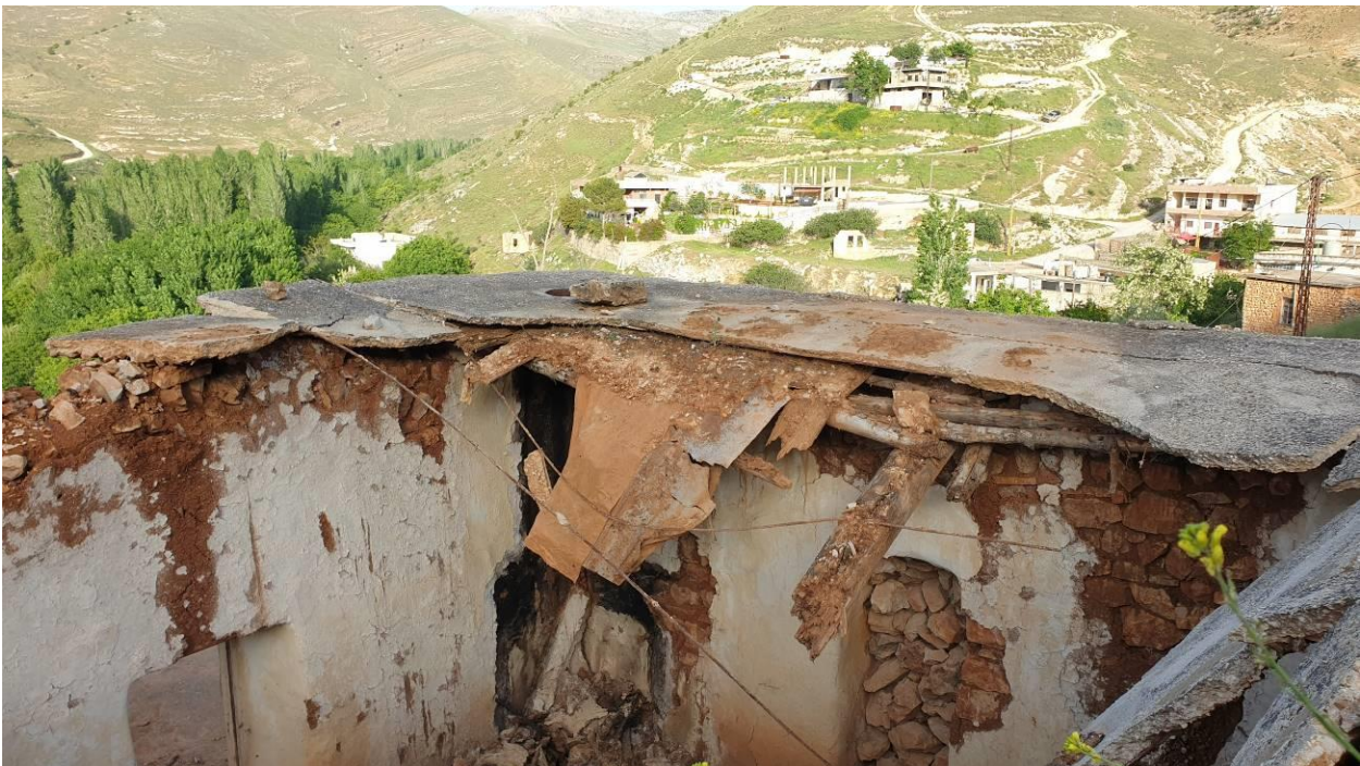
Figure 274 Fallen ceiling Yahfoofi - Bekaa Valley Source: Author (2020)
