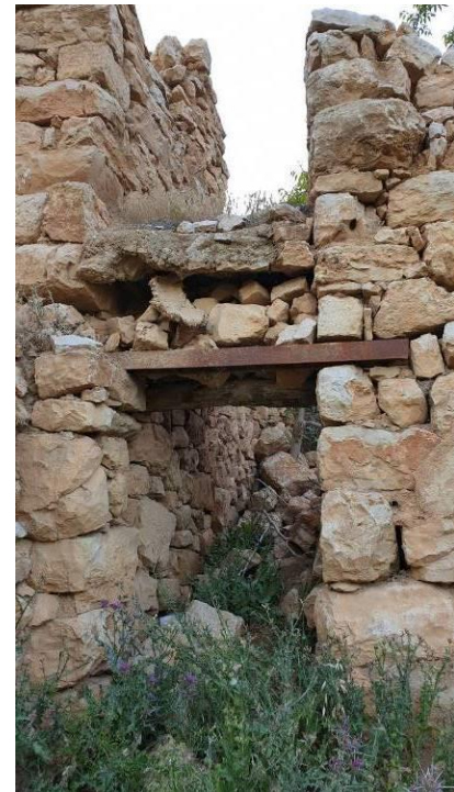
Figure 38 In the image above we see a dwelling in Yahfoufa – Bekaa, built during mid-19th century. Although the house is completely destroyed but the entrance wall and some of its walls still stand. On the entrance we can see an entrance door that had a wooden lintel, later on, during the late 20 th century, dwellers used the abandoned “railway” steel to use it as a lintel. In the image above we can see the wooden lintel at the back and then the entrance was modified by adding the steel bar from the old railway to hold the structure. Source: Author (2020)
