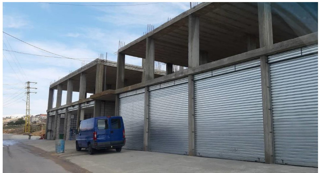
Figure 213 A street view of the construction. In the image above we see the 8 garages made. Source: Author (2018)
