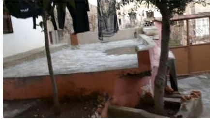
Figure 155 Old roof showing how it is finalized with concrete layer. Source: Author (2018)
