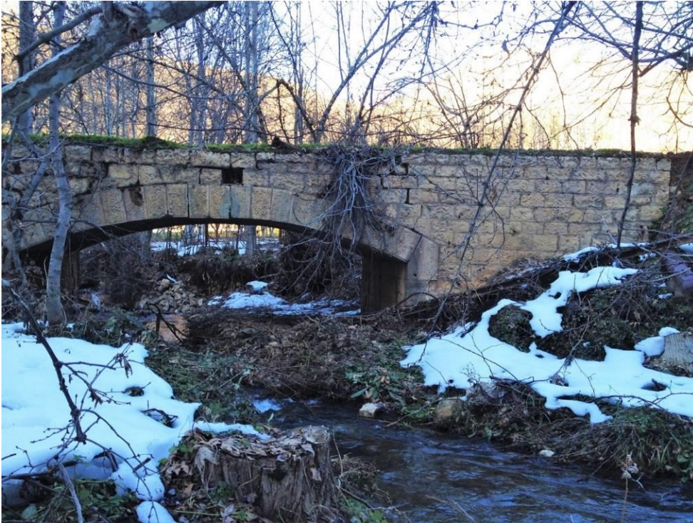
Figure 46 The old train's bridge over the Janta river made by during the French mandate. Source: Author (2018)
