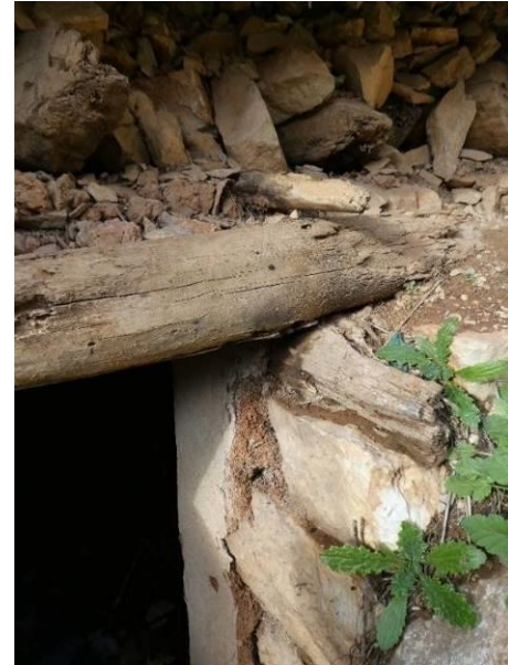
Figure 27 Construction detail of a vernacular dwelling in the Bekaa Valley Source: Author (2018)
