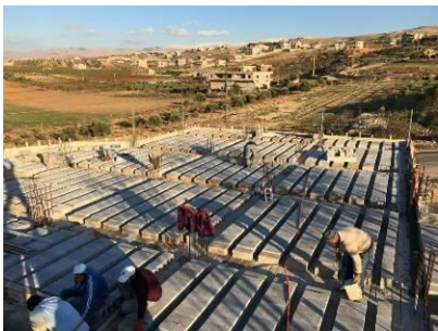
Figure 5 Roof slab concrete pouring during fall on the verge of winter Source: Author (2018)
