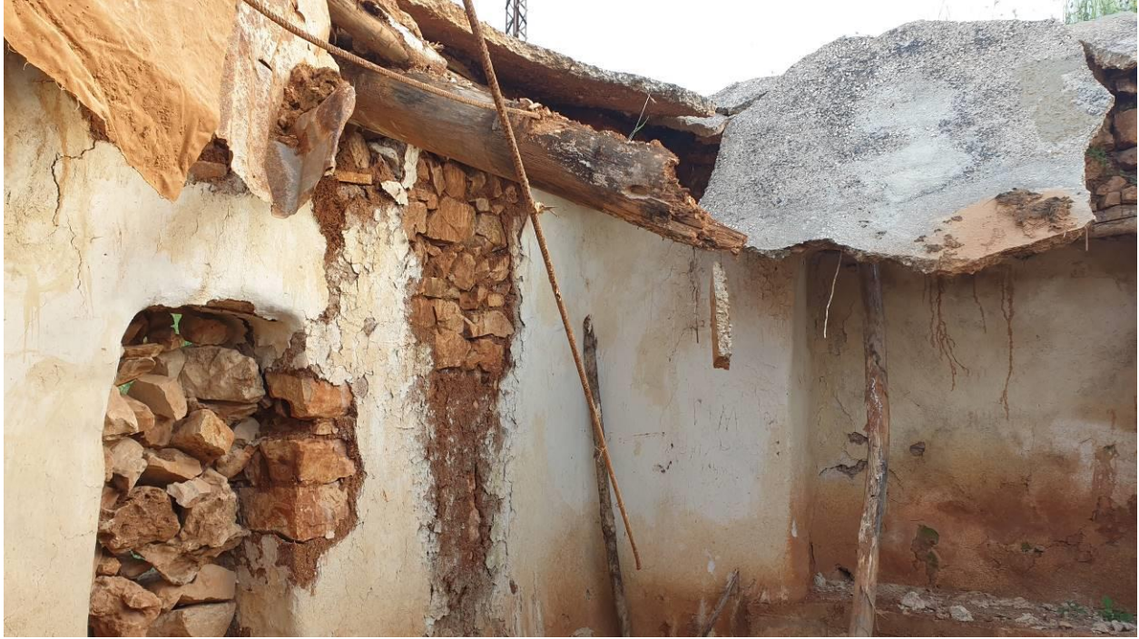
Figure 275 Interior of a destroyed house in Yahfoofa Source: Author (2020)
