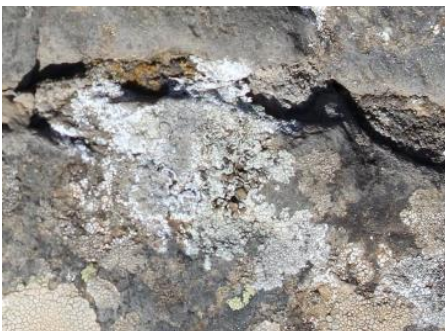
Figure 13. Efflorescence example from the site
