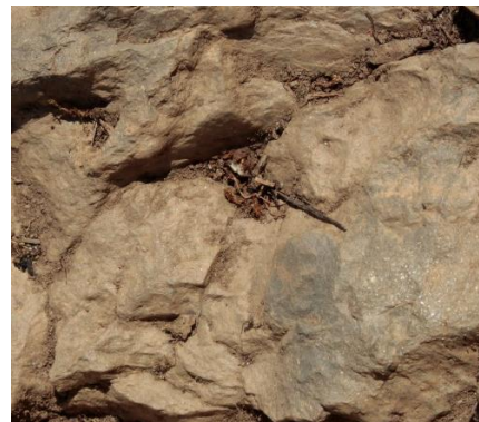
Figure 9. Differential erosion occurs when erosion does not proceed at the same rate from one area of the stone to the other. As a result, the stone deteriorates irregularly.
