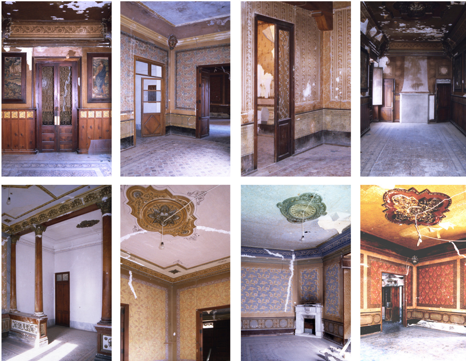
Fig 16. Casa de l'Hort (former Residence-Palace of the Cardinal Payá), Onil (Alicante, Spain), Feb-1996. Photographies of the Initial of the Building before its Drawing and its Rehabilitation. Photographs of the interiors of various rooms on the Main Floor (Noble Plan, Fig. 10). (Original Pictures: Martínez-Medina, A. & Sempere Valero, M.).
