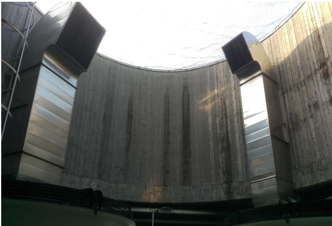
Figure 61. Technical floor over the second store, with the systems.
