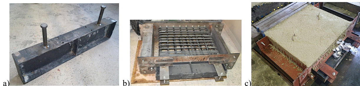
Figure 7. Specimen production. a) steel beam with welded headed stud anchors, b) reinforcement of the specimens and steel form, c) specimen after the concrete was poured.
