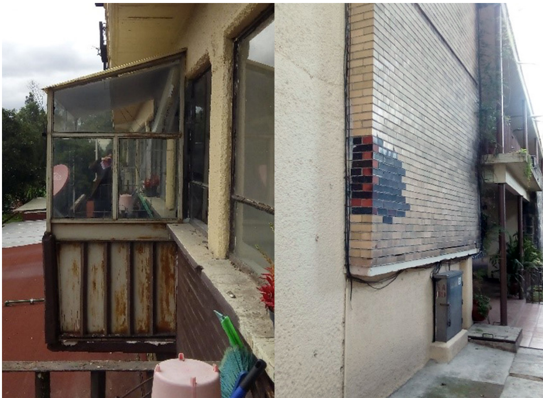
Figure 8. On the left, an enclosed balcony; on the right, painted bare materials and replaced un-matching glazed bricks, 2018.
