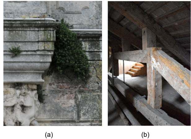
Figure 8: Detailed analysis of Villa Pisani external surfaces: a) Southern façade decay detail; b) roof system detail.
