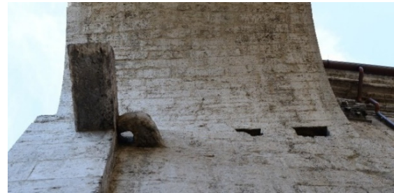
Figure 12: Detail of the stone corbel, belonging to a lintel, and of a stone hinge.
