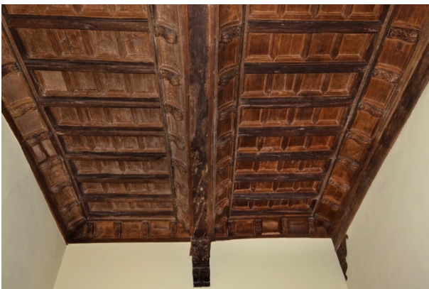
Figure 4: Timber floor from the late 15 th century, with corbels under the joists and concave bussole (photo by Giuliano Regis).
