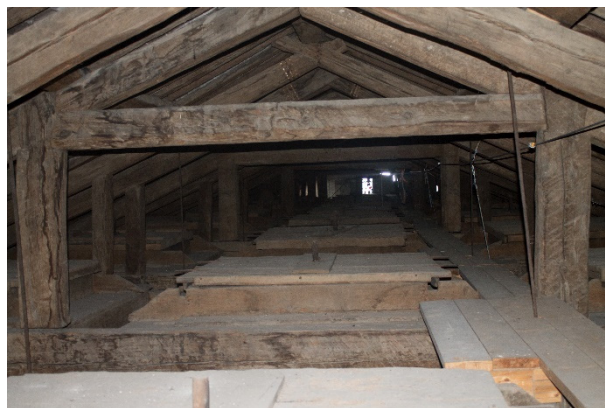
Figure 5: Photograph of the ceiling as seen from the attic; as is visible, the larger distance between the trusses is occupied by the coffer units.
