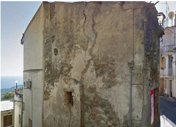
Figure 5: Image acquired by the drone relating to the identification of cracks.
