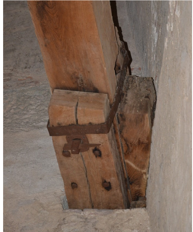
Figure 3: One of the metallic joints connecting the beams of the chestnut chain (photograph taken by the authors).
