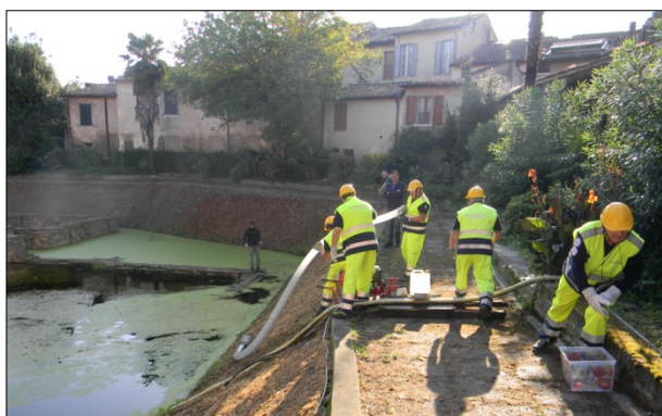
Figure 2: Draining operations of the area after the flooding event in August 2019.
