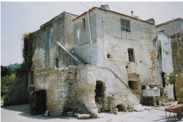
Figure 7: Tempio-Masseria del Gigante, Cuma. View of the north-west corner before the restoration work 1994, photos by R. Di Re.
