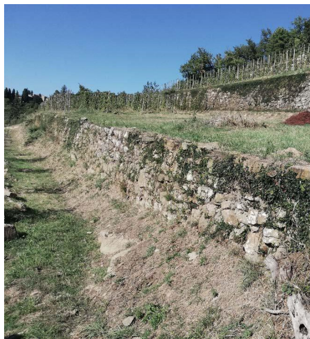
Figure 1: Dry-stone walls and terraces in the Grospoli II vineyard. Height of the dry-stone walls varies throughout the vineyard, as well as the distribution of the wine plants on each terrace.
