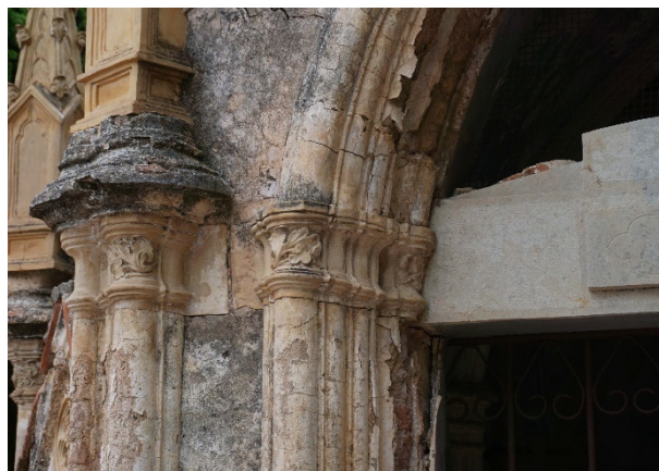
Figure 2: Some of the pathologies affecting the interior and exterior walls of the chapel.
