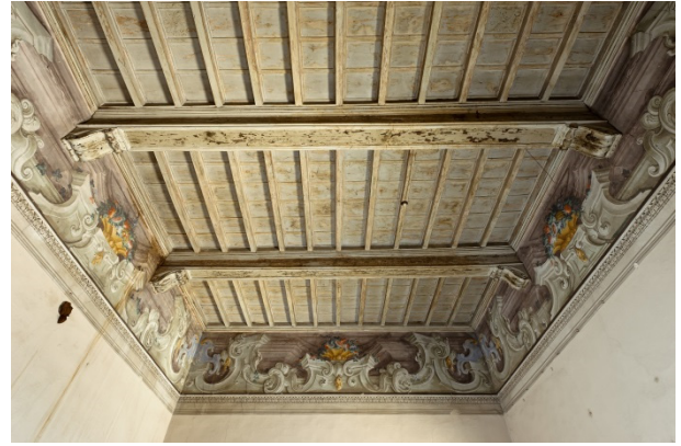
Figure 6: Timber floor with old girders; joists and planking were renewed between the late 17 th and the early 18 th centuries.
