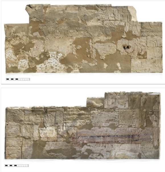
Figure 17: NW & NW Walls. The north west (top) and north east (bottom) walls of the Imperial Cult Chamber. Murray/The Epigraphic Survey 2017.
