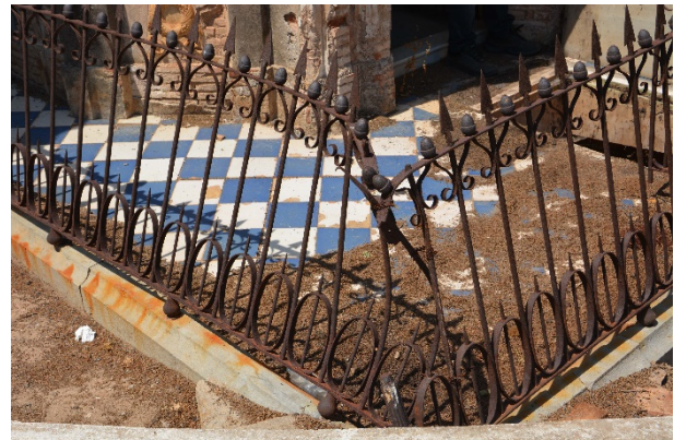
Figure 5: The northeast side of the iron enclosure with its deformation.
