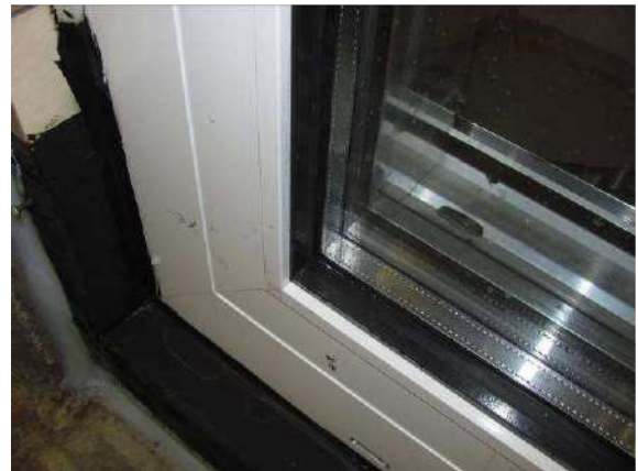
Photo 8 External sash, FR 2 at bottom lock side
