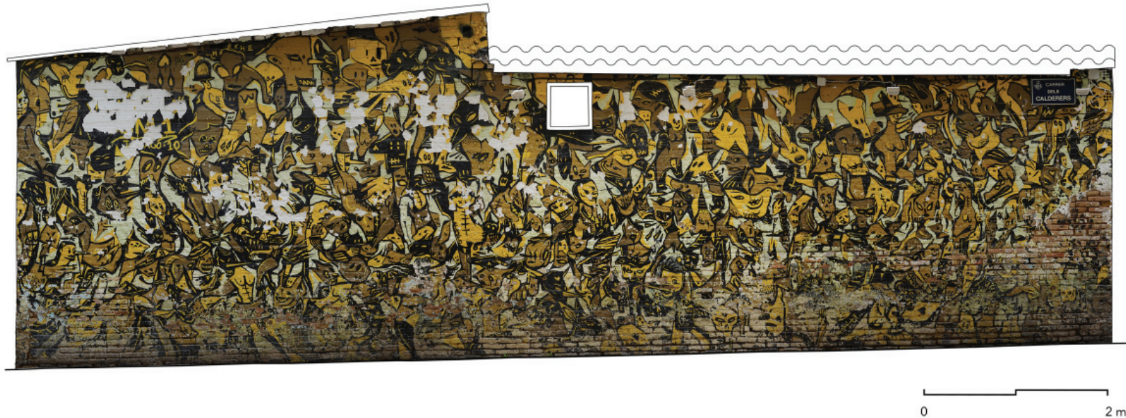
Fig. 10 - Graffiti Stop victim war's wall by Fasim. Photoplan obtained using photogrammetry SfM. Elevation facing Calderes St.
