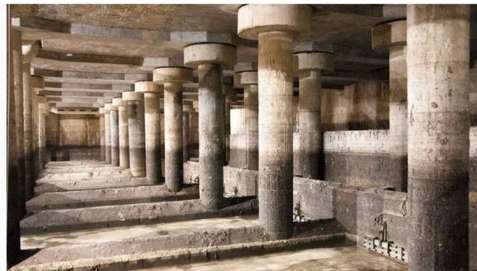
Figure 21. Example of an underground storm tank: Arroyo Fresno tank (Madrid). Source: Canal Isabel II, 2019
