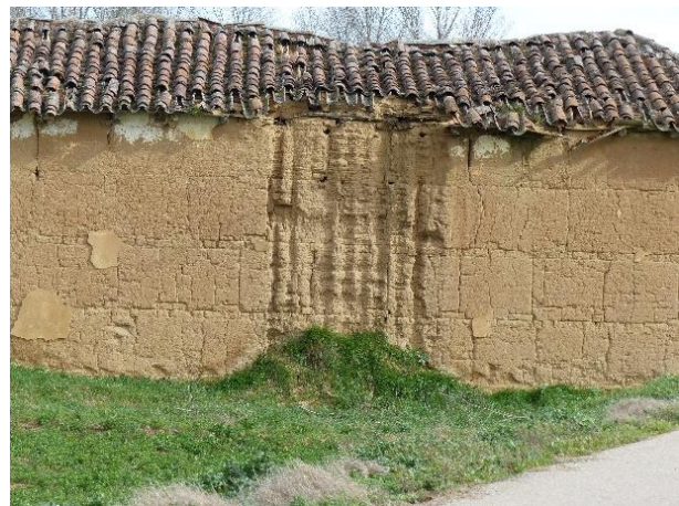
Figure 3. Washing of the wall caused by rain (Valderas, León)
