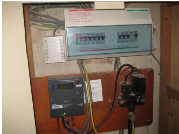
Figure 14 Electric Circuits and Meter
