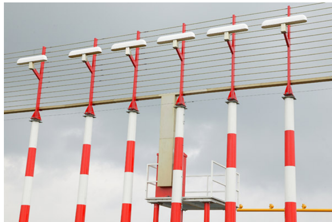
Figura 12. ILS Station on an airport, [6]
