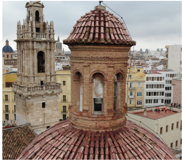
Figure 2: Detail view of the dome of the Santo Domingo Convent, Valencia for heritage inspection.
