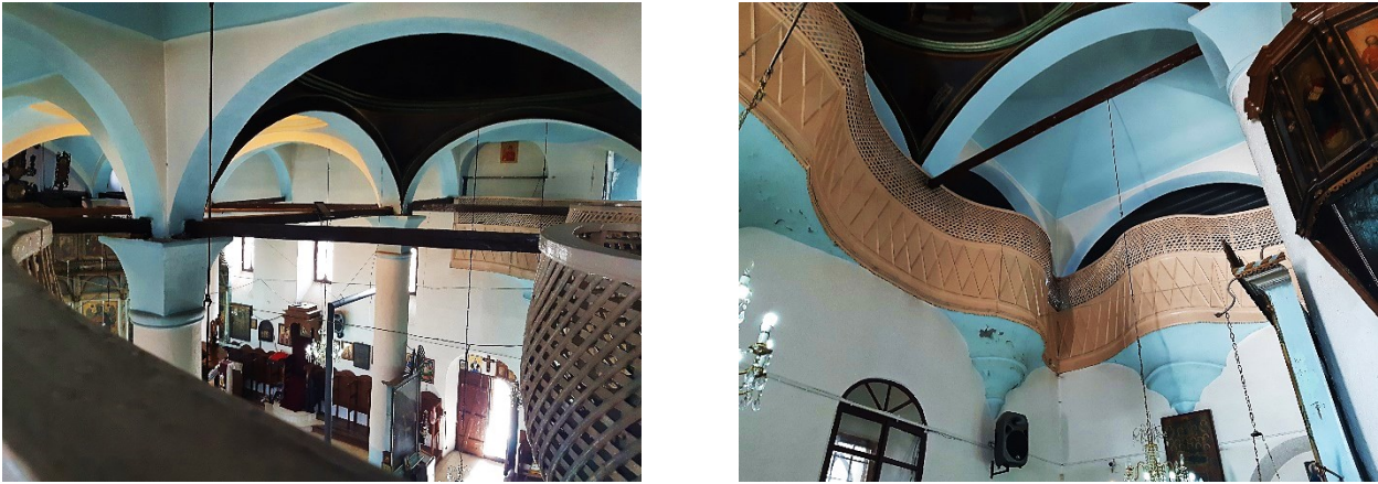
Figure III.238 Dormition of the Most Holy Mother of God in Krushevo: A. View from the northern gallery towards the south; B. View from the naos towards the north-west corner of the gallery.
