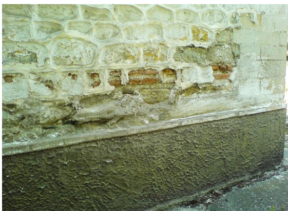
Figure III.224 St. Sunday in Bitola. Detail of the façade masonry of stone and brick layers, disguised with protruding mortar joints.
