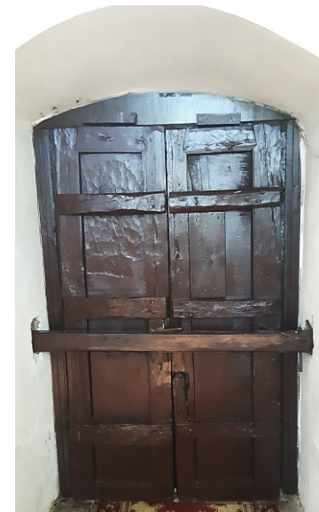
Figure III.190 St. George in Drmeni (Prespa). Internal view of the west entrance portal.
