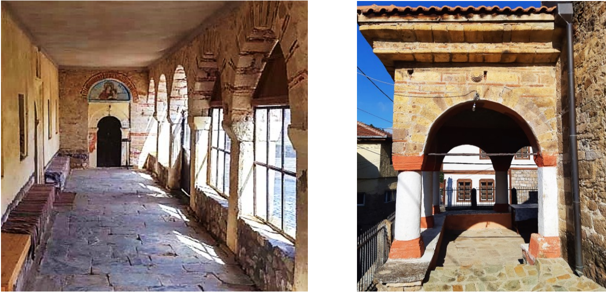
Figure III.50 A. St. Demetrius in Magarevo (Bitola); B. St. John in Kratovo. View of the masonry open porches.
