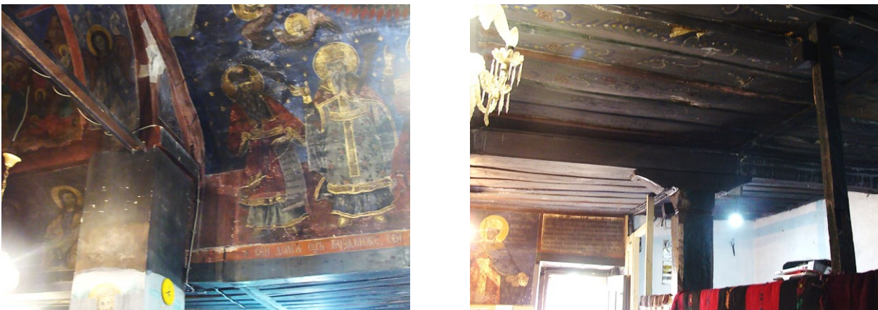
Figure I.47 St. Nicholas in Gluvo (Skopje). A. View of the remaining southern pillar where the post-Byzantine masonry vault and the Revival false vault meet; B. View towards the narthex and the entrance to the naos.
