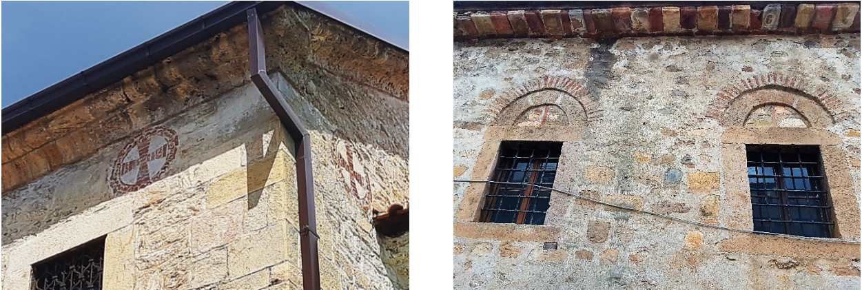
Figure III.96 Details of façade decoration in brick: A. St. George in Resen; B. St. John in Kratovo.
