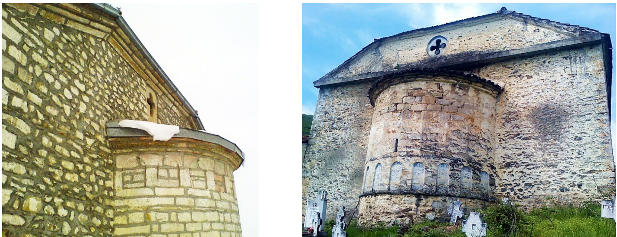
Figure III.29 Examples of altar apses with a frieze of blind arched niches. A. St. George in Logovardi; B. St. Nicholas in Dragosh, both in the region of Bitola.
