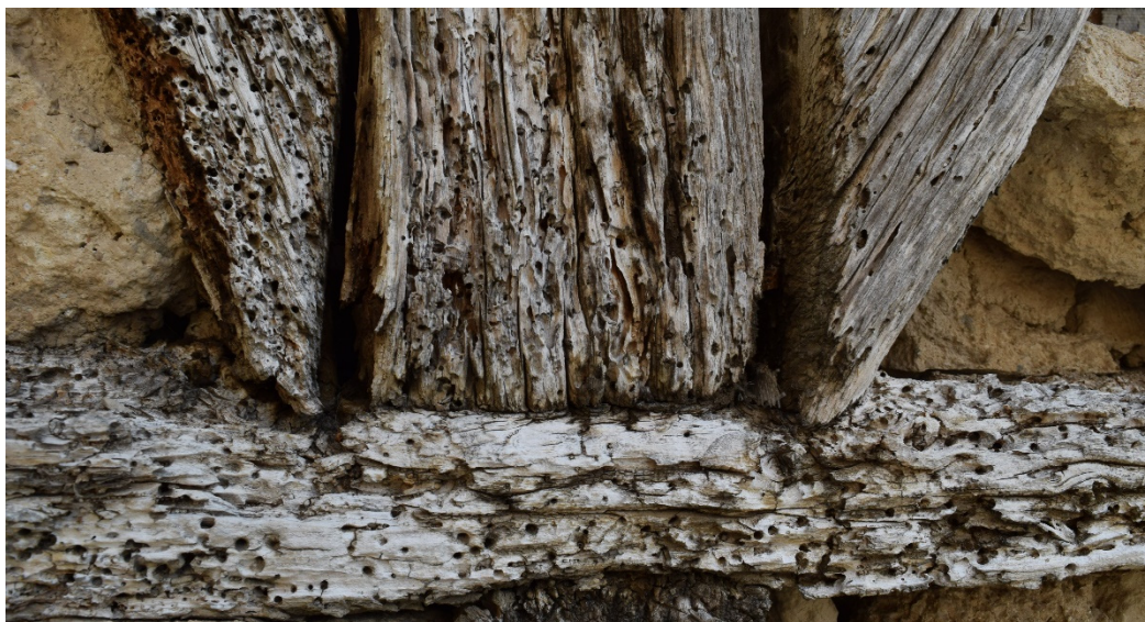
Figure 21. Attack by xylophagous insects at the meeting of wooden elements where moisture accumulates, in a half-timbered wall in Valdazao (Burgos).
