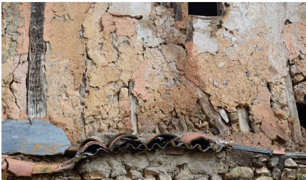
Figure 16. Chipping and gaps in the lime or gypsum mortar rendering of a half-timbered wall in Santibañez de Ayllón (Segovia).
