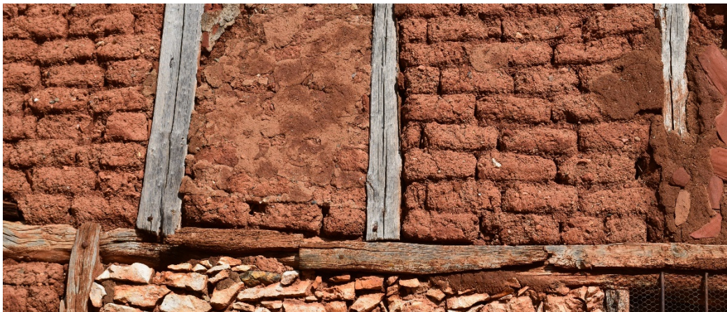
Figure 8. Different degrees of erosion in a half-timbered wall in Ayllón (Segovia).
