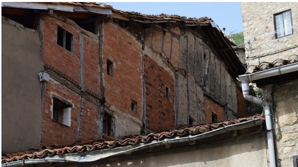
Figure 25. Replacement of the monolithic traditional filling with industrial brick and modifications of the timber structure, in a half-timbered wall in Pancorbo (Burgos).
