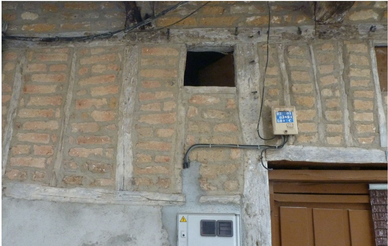
Figure 30. Rejoint of a fabric filling of a half-timbered wall in Garganta la Olla (Cáceres).
