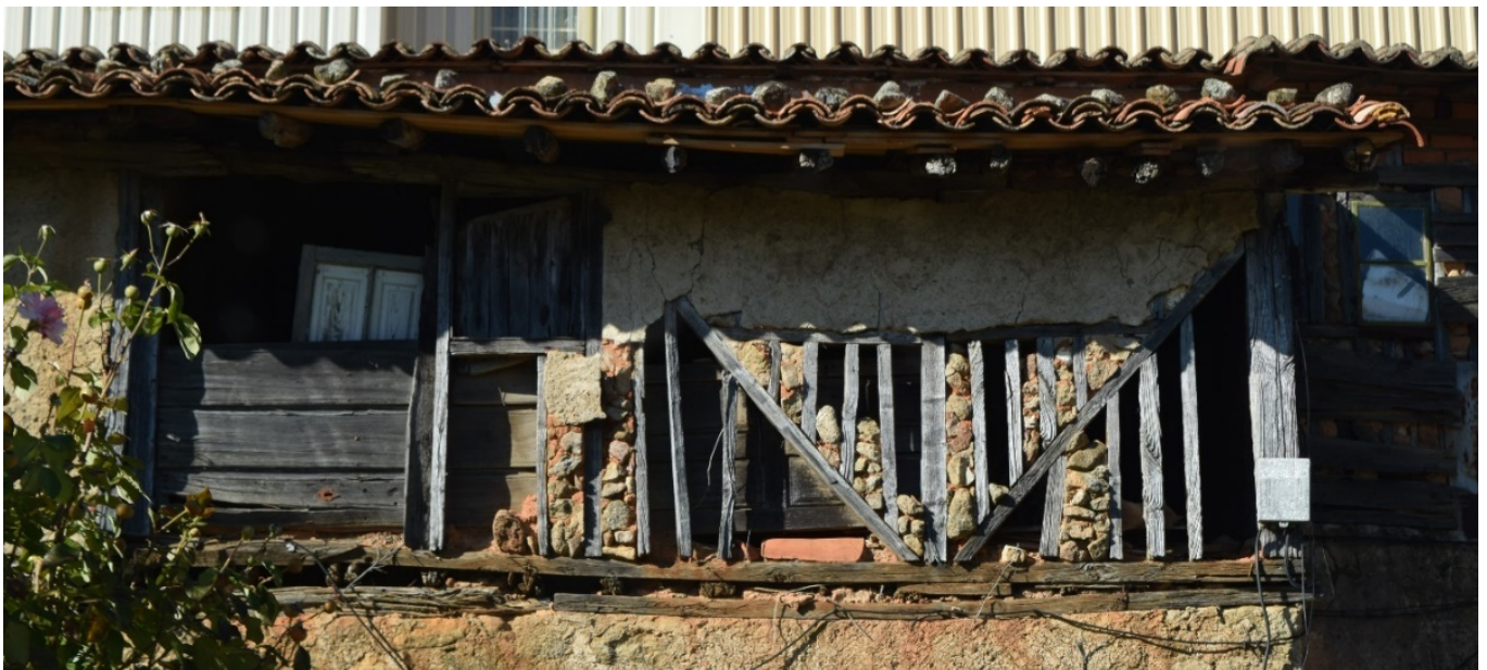
Figure 10. Volumetric loss of the monolithic filling of a half-timbered wall in Cepeda (Salamanca).
