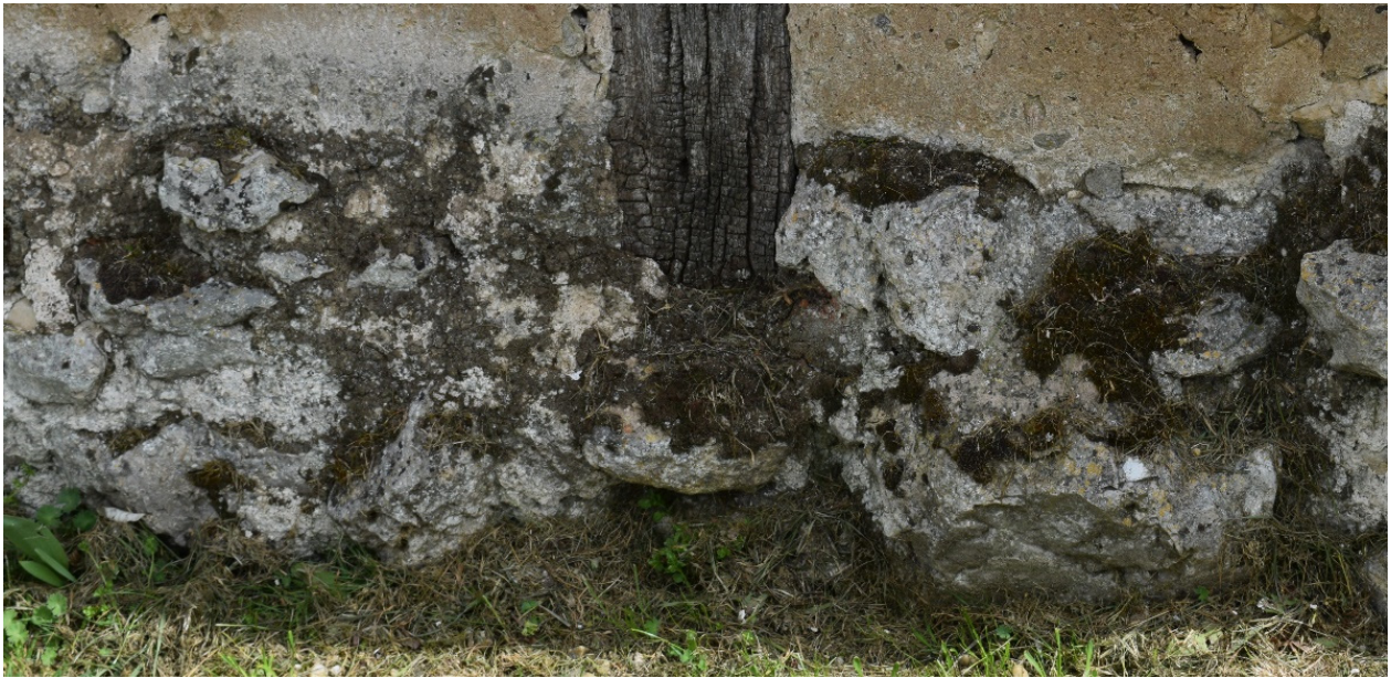
Figure 23. Cubical brown rot in the lower part of a pillar in contact with the humidity of the ground, in a half-timbered wall in Ages (Burgos).
