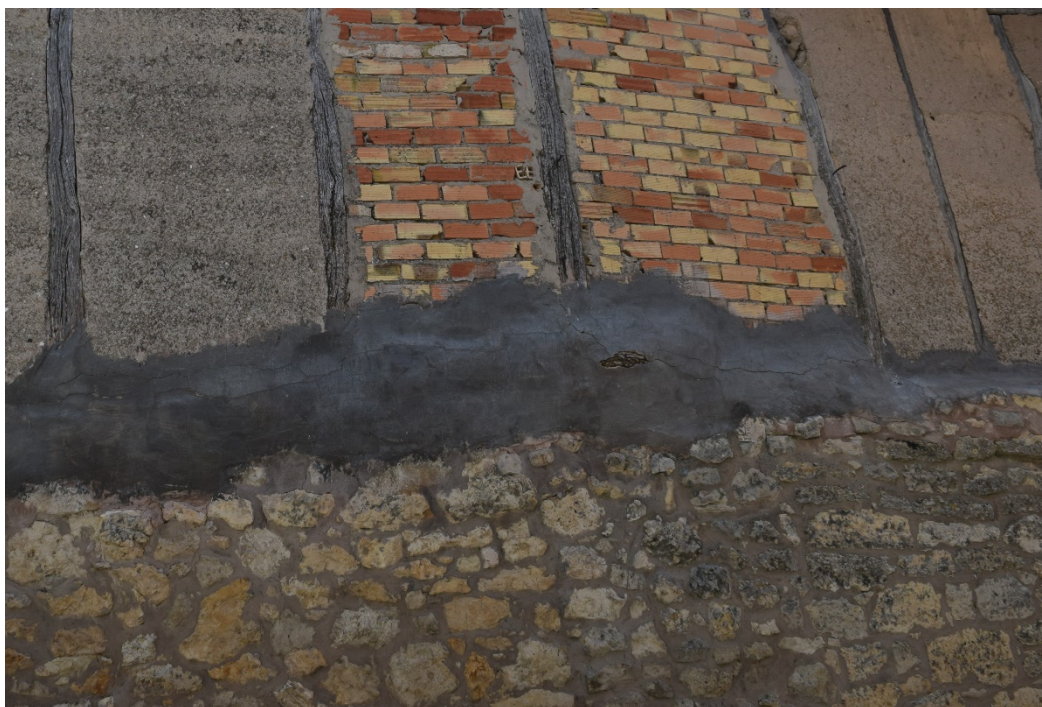
Figure 7. Efflorescence on a half-timbered wall in Reinoso (Burgos), where concrete mortar has been used to repair the encounter with the lower wall.
