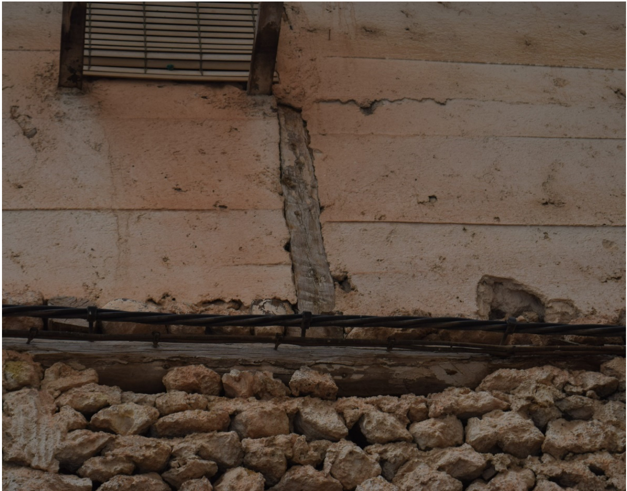
Figure 29. Cables installed following the geometry of the timber structure in a half-timbered wall in Santa Cruz de Moya (Cuenca).
