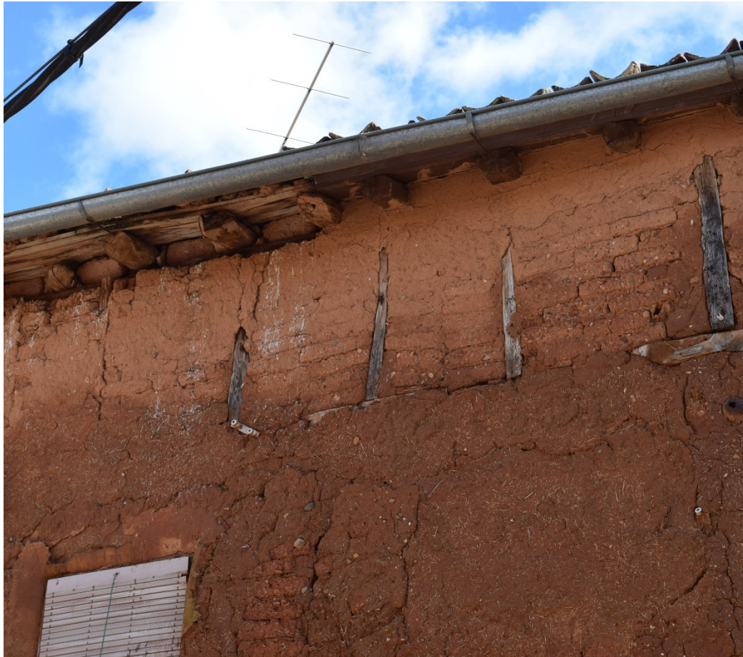
Figure 4. Damp stains in the lower part of a half-timbered wall in Ayllón (Segovia), where the eaves do not protect from the incidence of rain.
