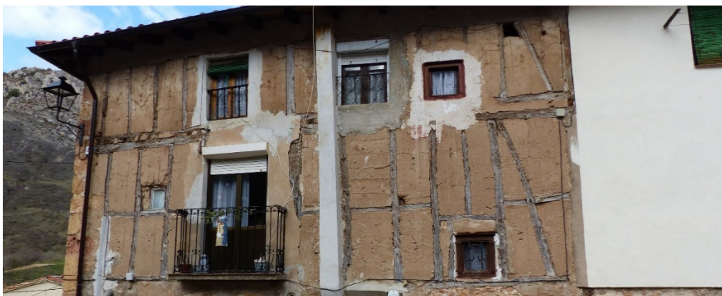
Figure 26. Addition of openings and installation of unsuitable elements such as shutter boxes and ventilation chimneys in al half-timbered wall in Poza de la Sal (Burgos).
