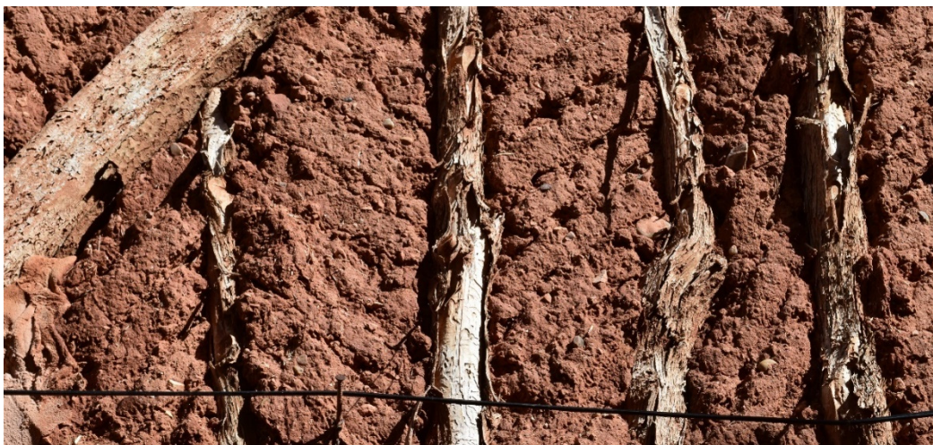
Figure 14. Significant deterioration of the wood cracks in a half-timbered wall in Ayllón (Segovia).
