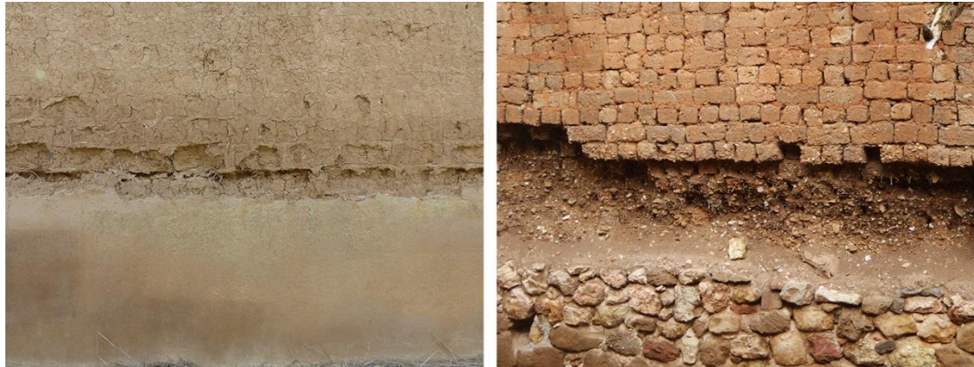
Figure 7. Superficial (left) and volumetric (right) erosion due to rising damp.
