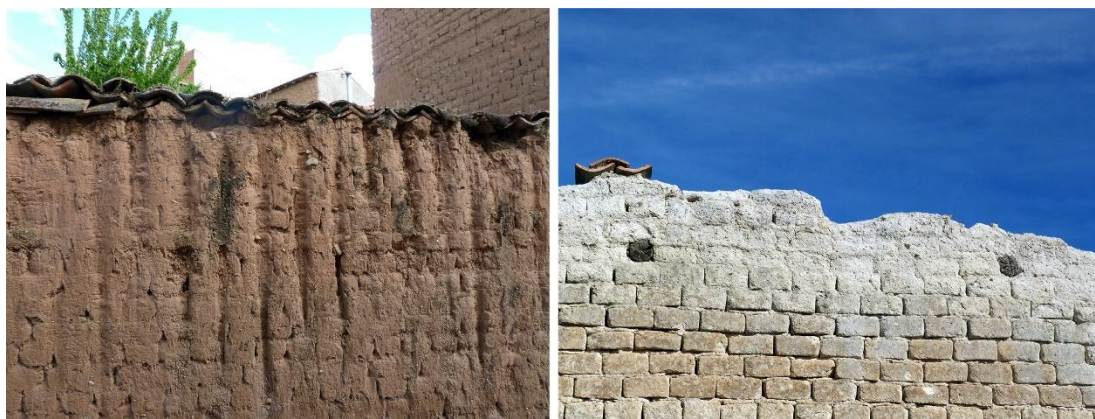
Figure 10. Superficial (left) and volumetric (right) erosion due to washing.
