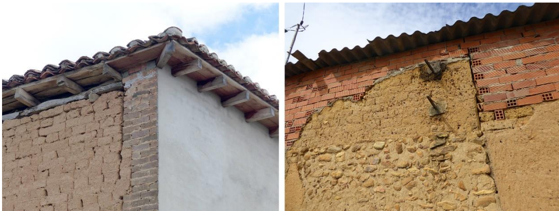
Figure 17. Cracks due to lack of interlocking between constructive elements.
