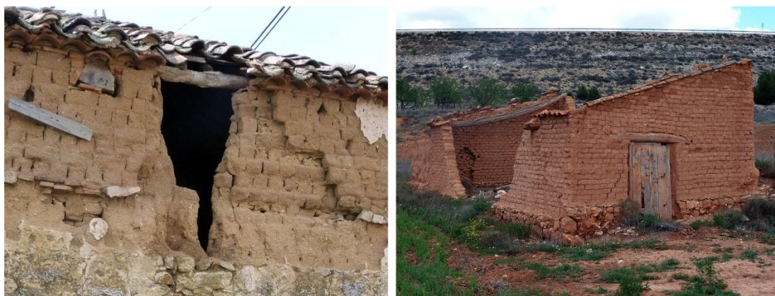
Figure 12. Localised (left) and complete (right) loss of the roof and subsequent collapse of the wall.
