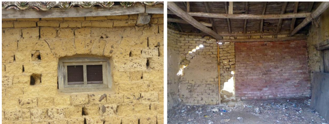
Figure 15. Cracks due to structural weakness introduced by openings.
