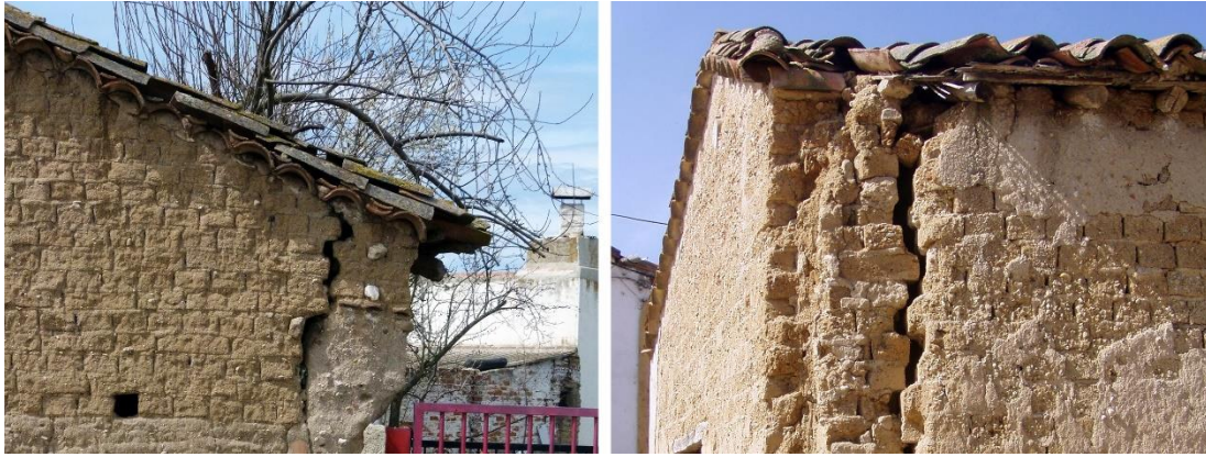
Figure 16. Cracks due to wall rotation from roof thrust.
