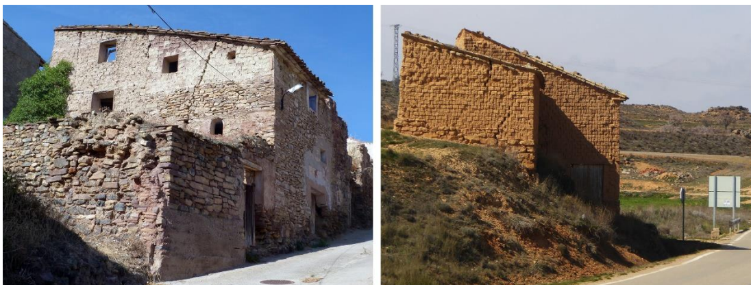
Figure 18. Cracks due to foundation failure.
