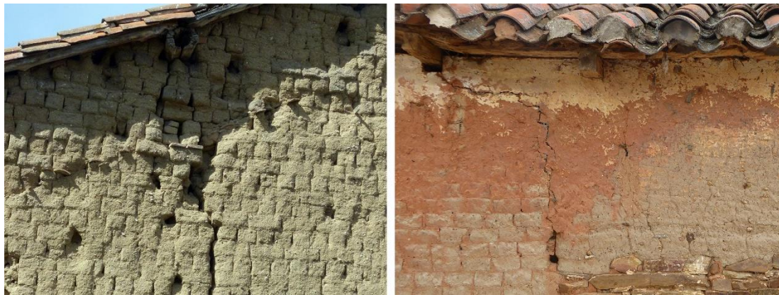
Figure 14. Cracks due to concentrated loads introduced by beams.
