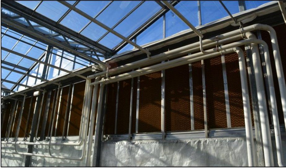
Figure 3.3 - Evaporative pads installed in the monitored greenhouse.
