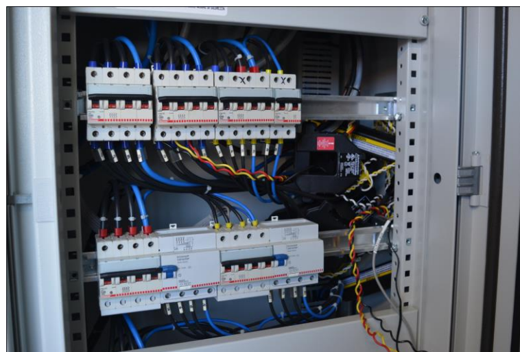
Figure 3.16 – Detail of the electrical panel with the kW-transducer connected.
