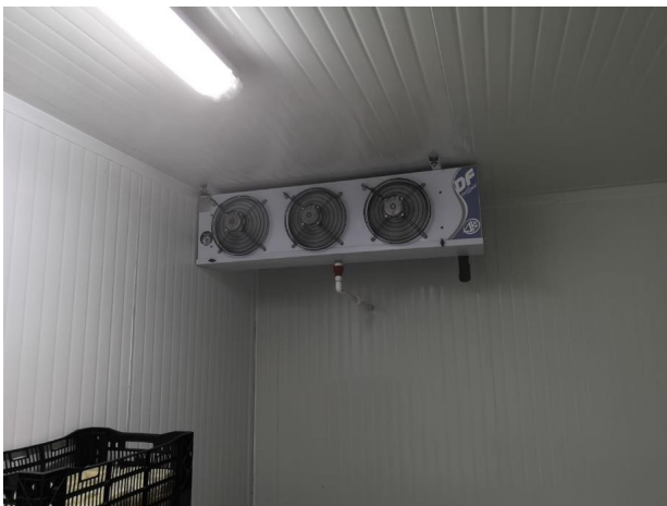
Fig. 5. Cold Room with Ventilation.
