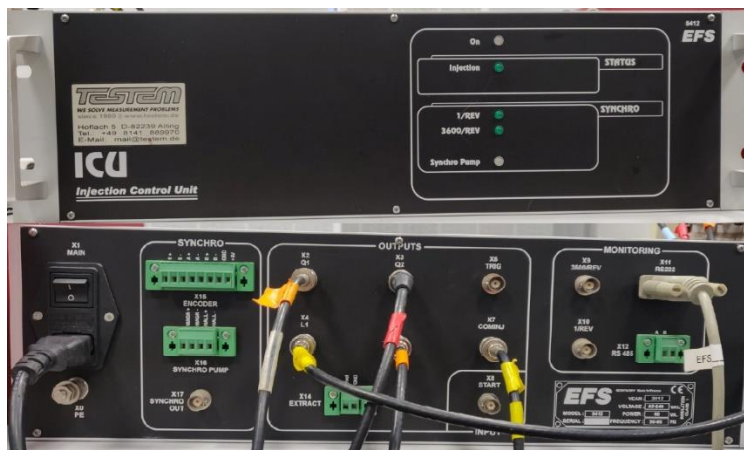
Figure 4.3 Injection Control Unit ICU
