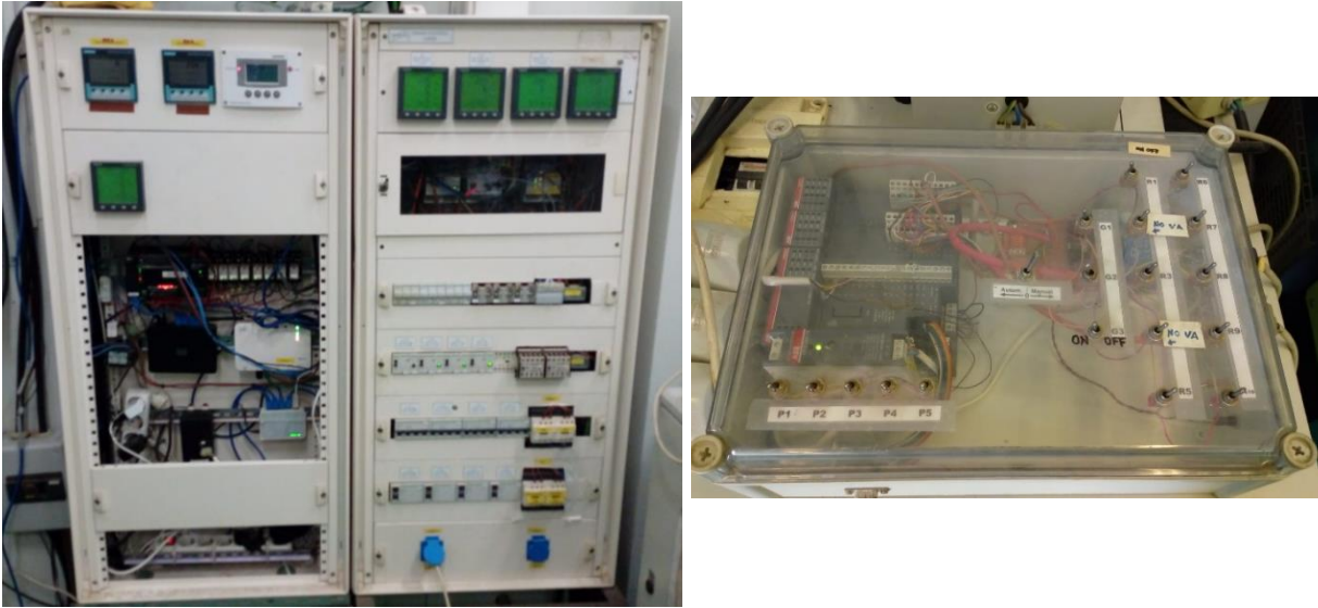
Figure 8. Control elements from labDER HRES. (a) Protection and measurements system. (b) Programmable load.
