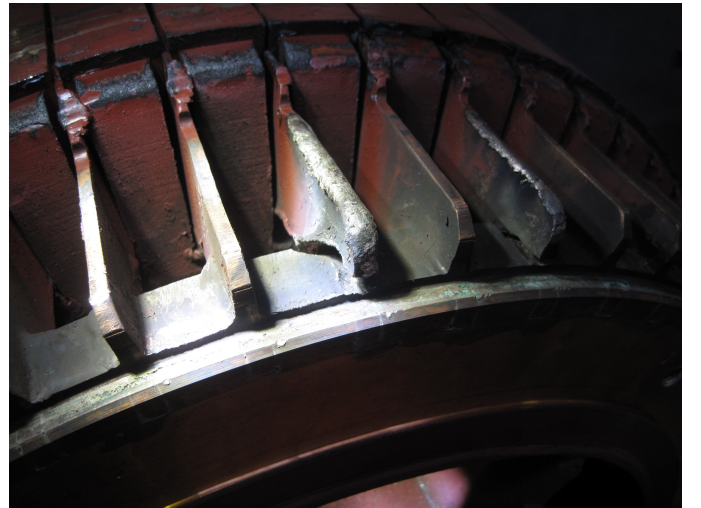
Fig. 1. Motor of Appendix A (3.15 MW), with a broken bar fault.
