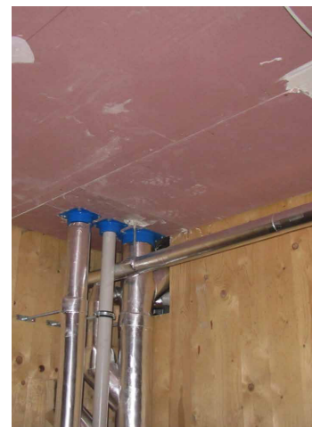
Imagen 2.95 Panel perforado e instalaciones hidráulicas. - Forté – Building, australias first timber Highrise, Lend Lease and WoodWorks
