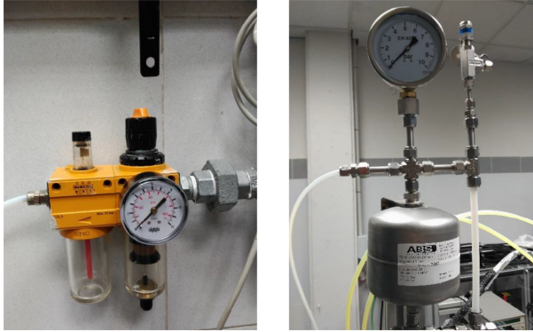
Figure 3.20: Pressure gauges employed in the installation.
