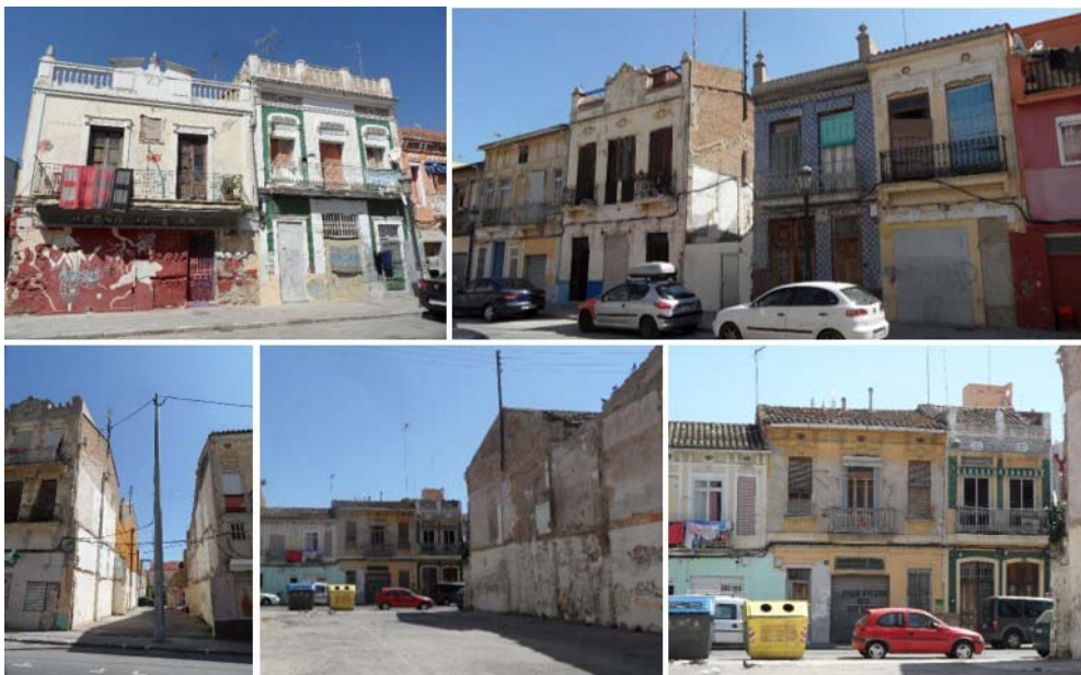
Figure 5. Example of residential buildings in Ground Zero Area with a bad state of maintenance, ruined buildings and empty plots (credit: the authors)
