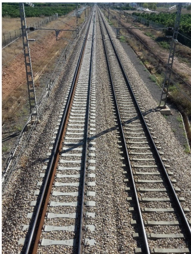
Fig. 1. Conventional railway track (right) and dual gauge track (left) in Spain.
