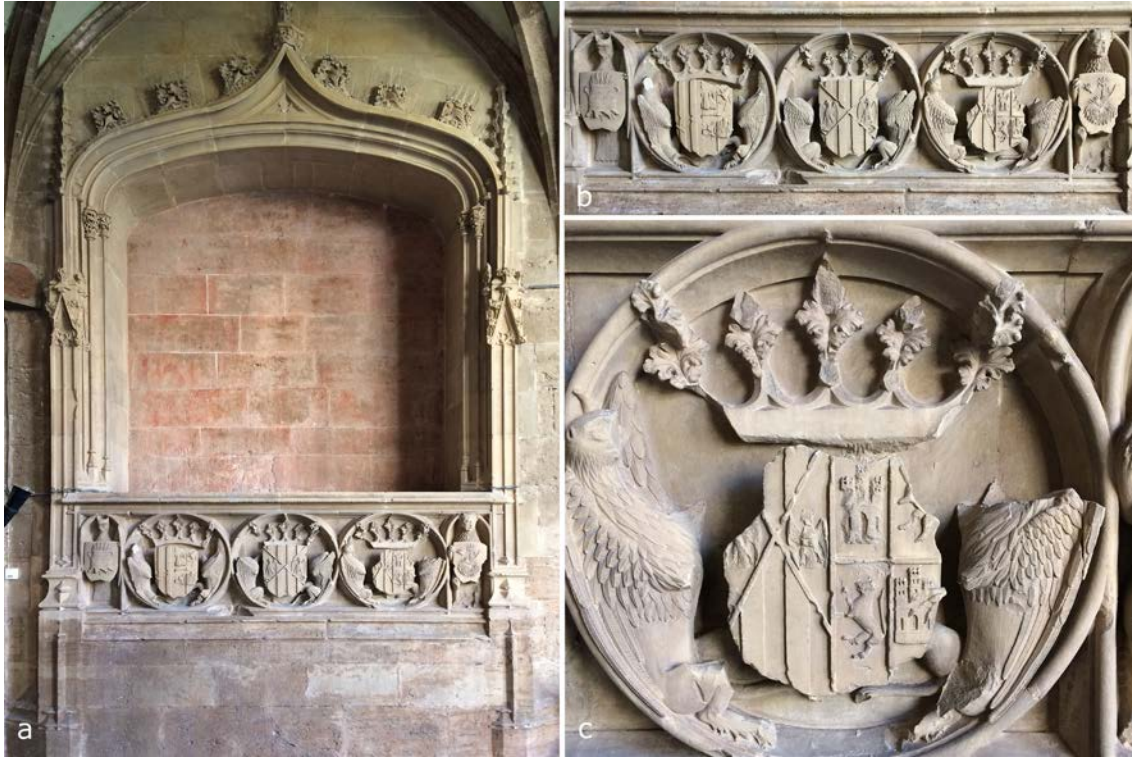
Fig. 1 (a-c). The Stone Sepulcher of the Queen Mary of Castile”, Royal Monastery of the Holy Trinity (Valencia, Spain). a) General view of the Sepulcher; b) Zones of the tondos where it observes the coats of arms damaged; c) Detail areas of the missing sections of tondo where the study is applied.
