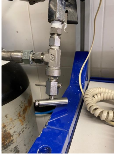
Figure 9.18: Closing of Purge Valve
