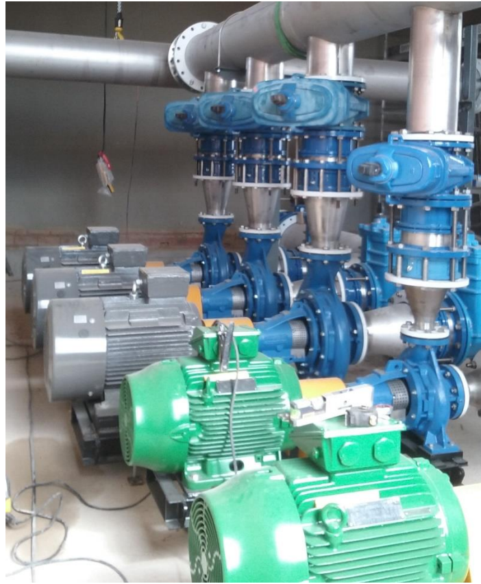
Figure 6: Pumping system for the new Mareny de Barraquetes reservoir
