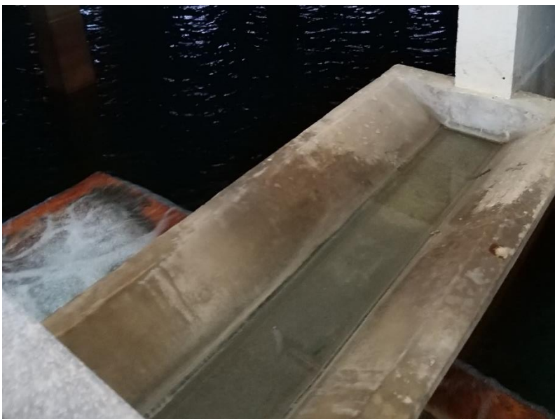
Figure 10: Evacuating vessel and sand traps
