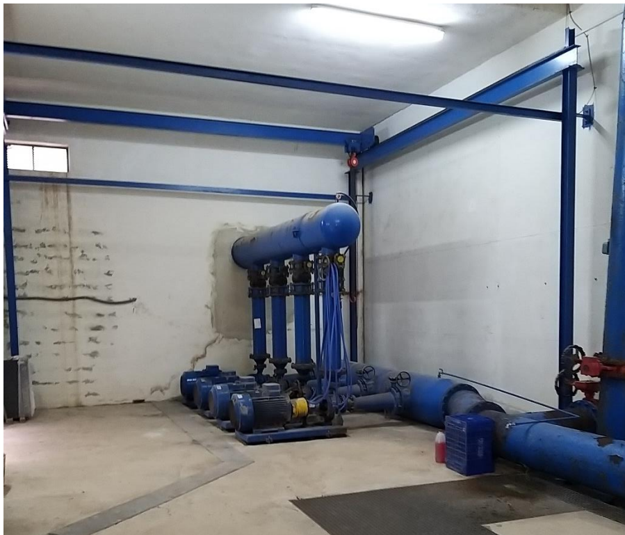
Figure 13: La Malva pumping system
