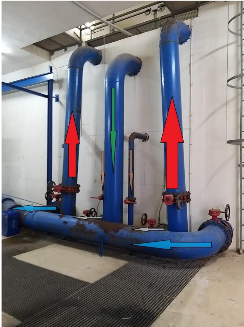
Figure 9: Inlet and outlet pipes in La Malva reservoir
