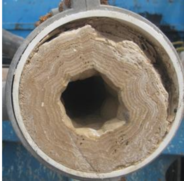
Figure 51: Pipeline with extreme case of sedimentation
