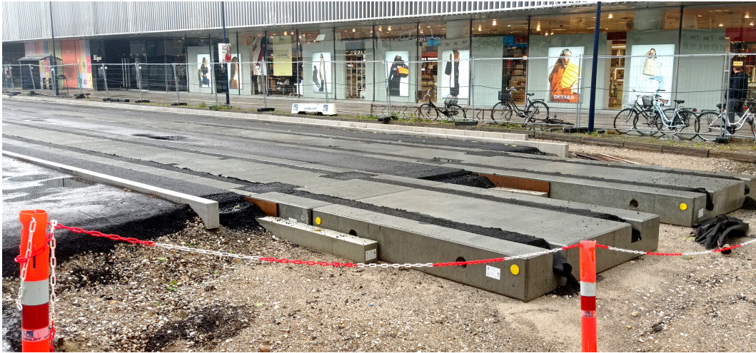
Figure 1.3: Laying of precast concrete slabs that are part of the track of the Ring 3 light rail line on the section next to the Lyngby shopping center.
