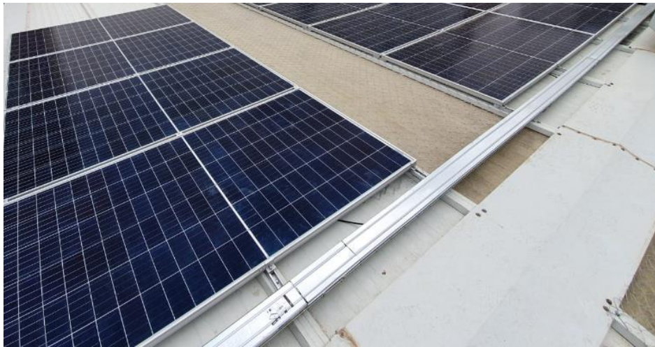
Figure 89. Photograph of an example installation showing the attachment to the ribbed roof. Source: Own.
